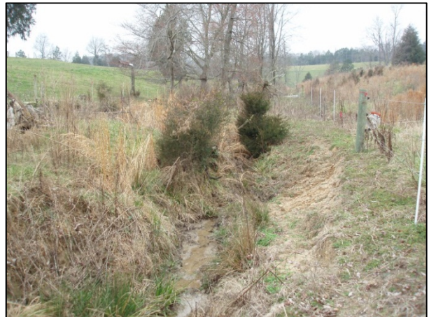
Looking downstream at cattle damage on T1A-1. 2/10/2012
