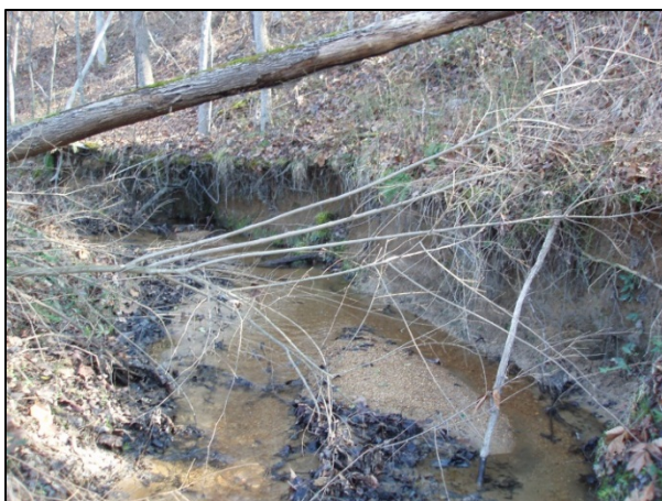
Looking upstream at an eroded bank on T2-1. 2/10/2012
