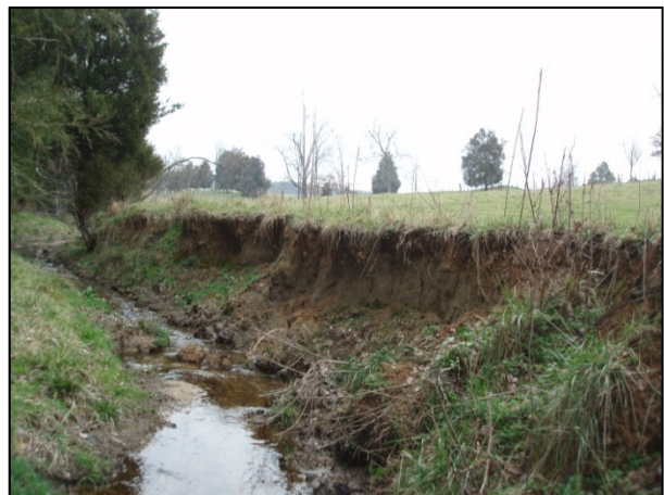
Looking upstream at degraded bank on T1-2. 2/10/2012
