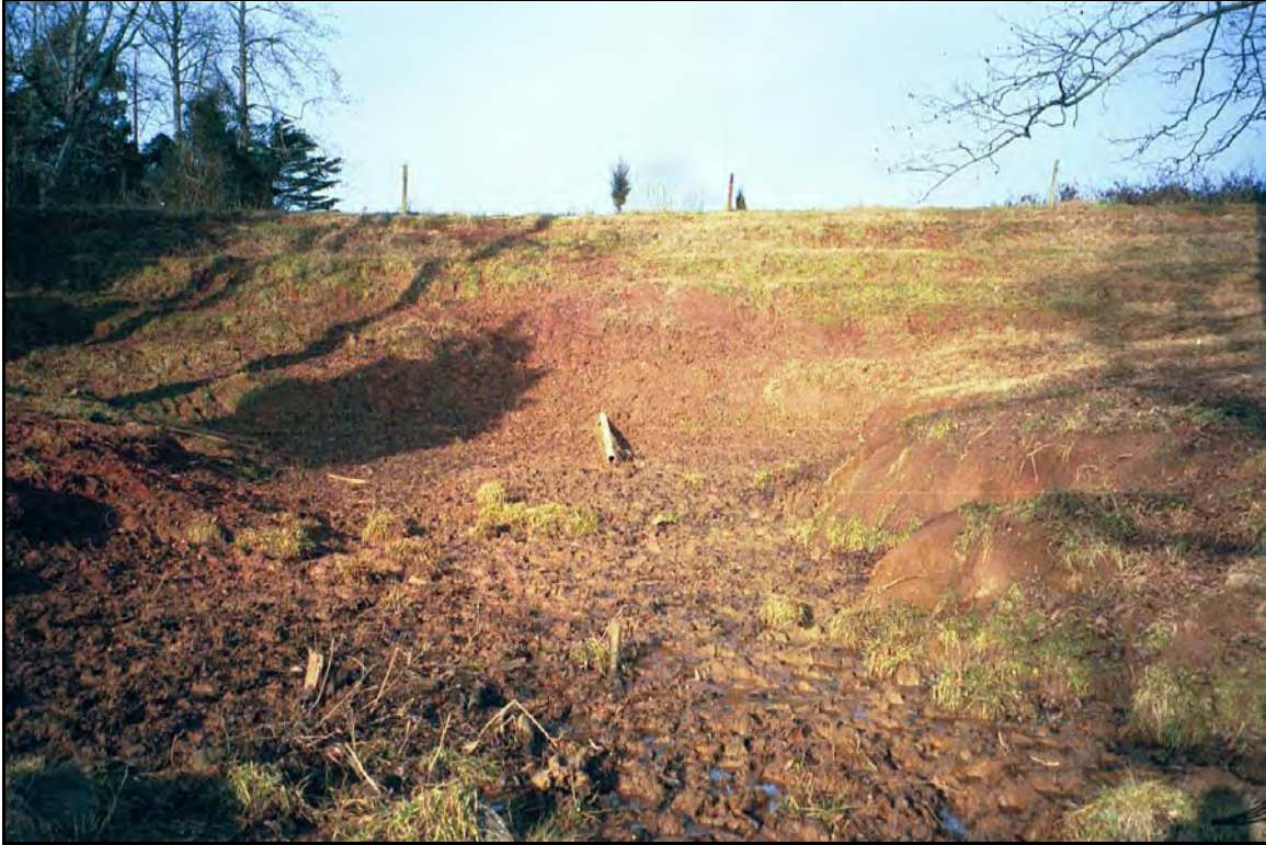
Photograph 7 – Four-inch PVC pipe drains water from pond into UT2.
