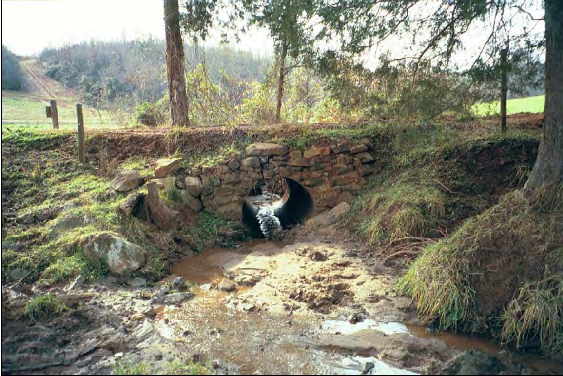
Photograph 17 – Forty-eight inch CMP conveys stream flow under dirt road leading to the northwest portion of the Johnson property.
