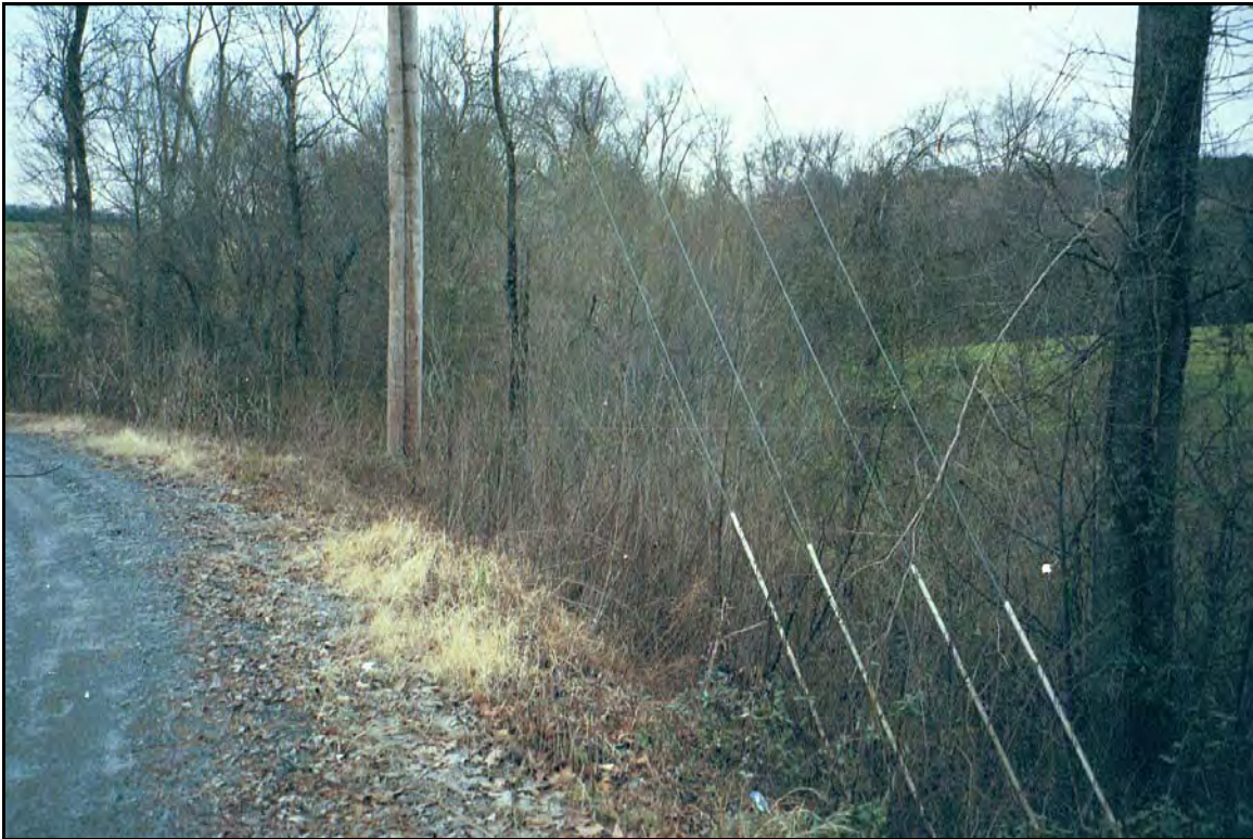
Photograph 26 – Power poles and guy wires adjacent to the south bank of UTLHC. Locations are approximated on Figure 5 – Existing Conditions.
