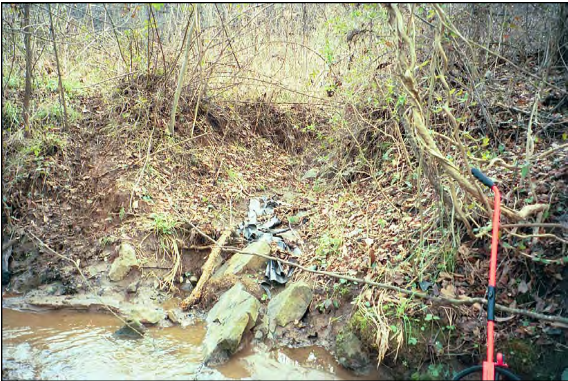
Photograph 22 – Roadside drainage from Hunting Creek Road drains to UTLHC via rock lined channel.
