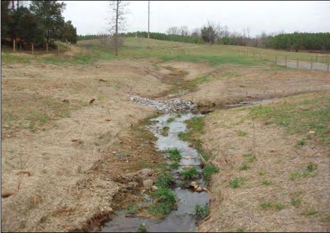
Photo Point 5a: View looking upstream towards Tributary 2 on main stem near Station 12+50. 12/13/07 – As-Built
