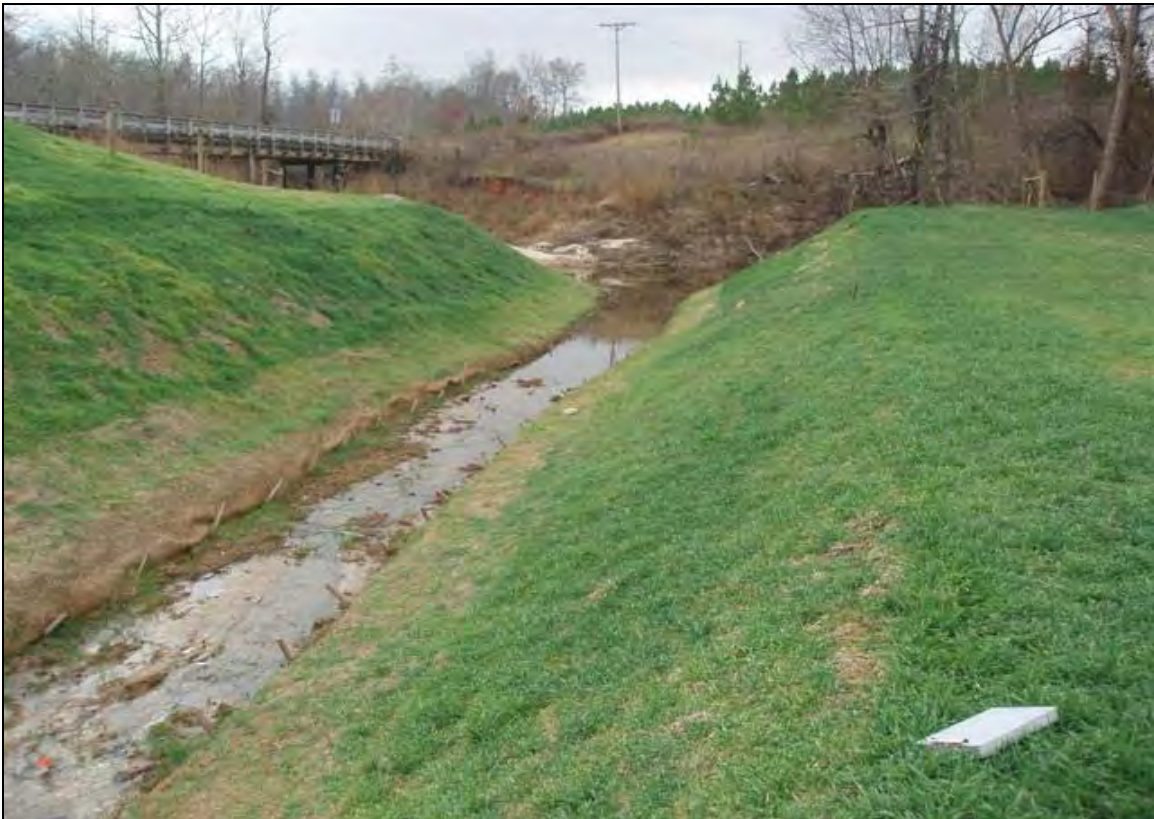
Photo Point 12b: View looking toward confluence with Little Hunting Creek. 12/13/07 – As-Built
