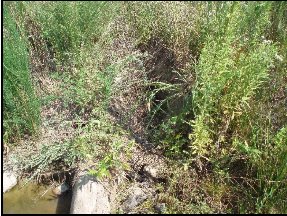
SPA 3. UT1. STA 20+20, heavy erosion on right bank, endcut around log grade control, small gully located immediately downstream of grade control.
