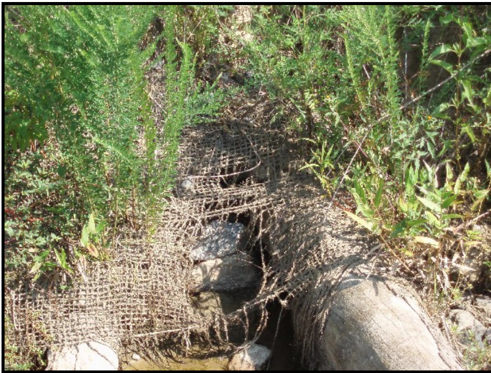
SPA 4. UT1. STA 20+20, erosion occurring around log grade control.
