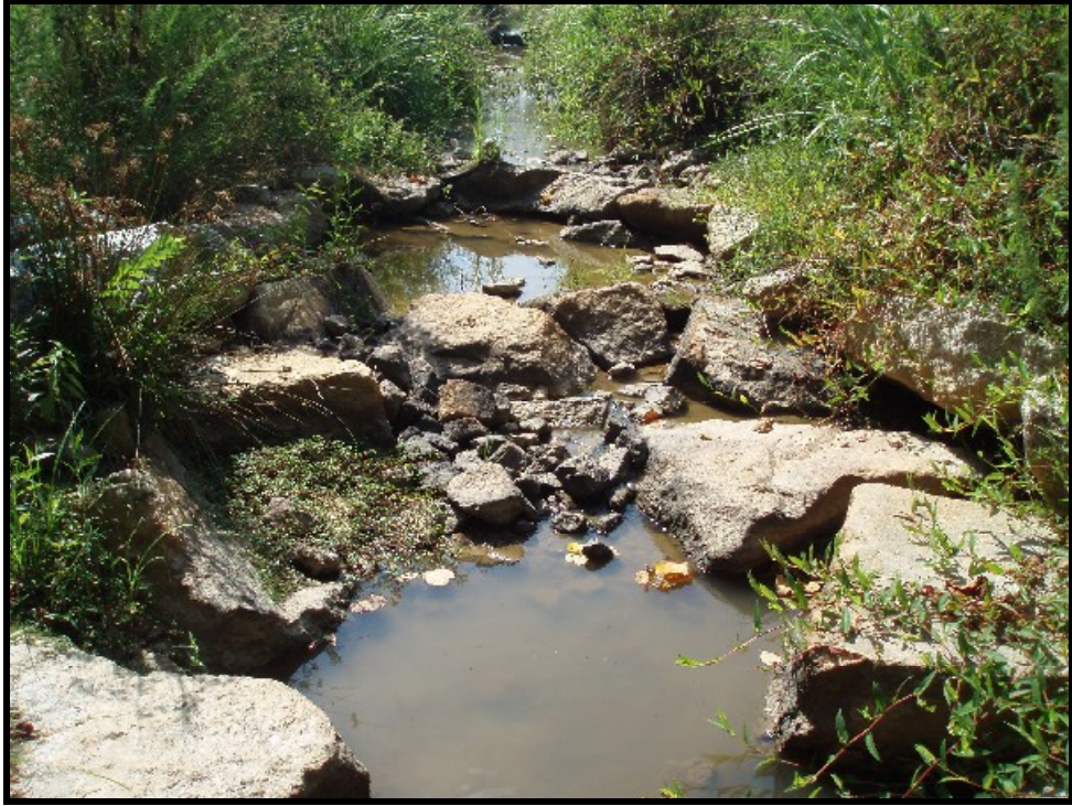
SPA 5. UT1. STA 22+00, rock cross vane short cut around header rock, no erosion.
