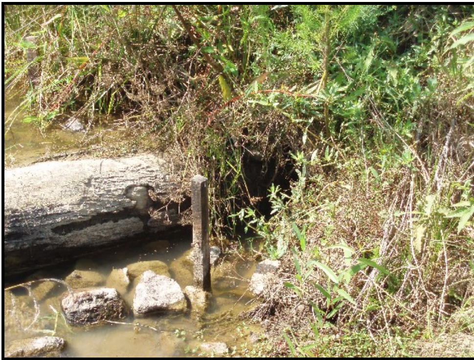
SPA 2. UT1. STA 18+90, erosion on left bank downstream of grade control, downcutting downstream of log has perched log.
