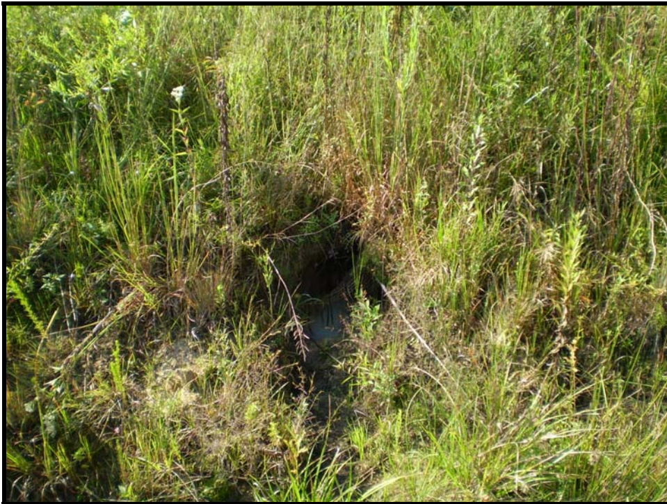
SPA 2, UT1 Station 20+50 – Left bank erosion; headcut
