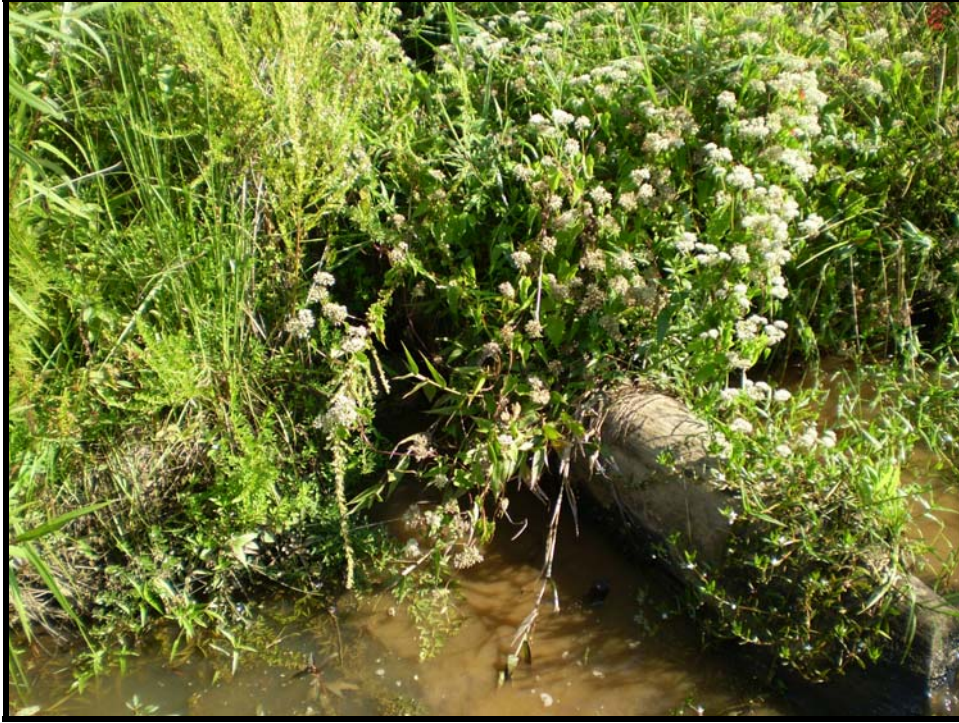
SPA 1, UT1 Station 20+25 – Log weir washed out
