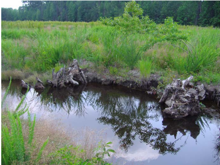
Photo 8. Example of eddies that have caused scouring and erosion around the toes and banks of the root wad structures (7/4/07)
