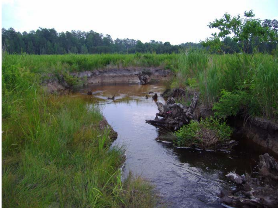
Photo 1. Looking downstream at the start of the head cut at Station 33+00 (7/4/07)
