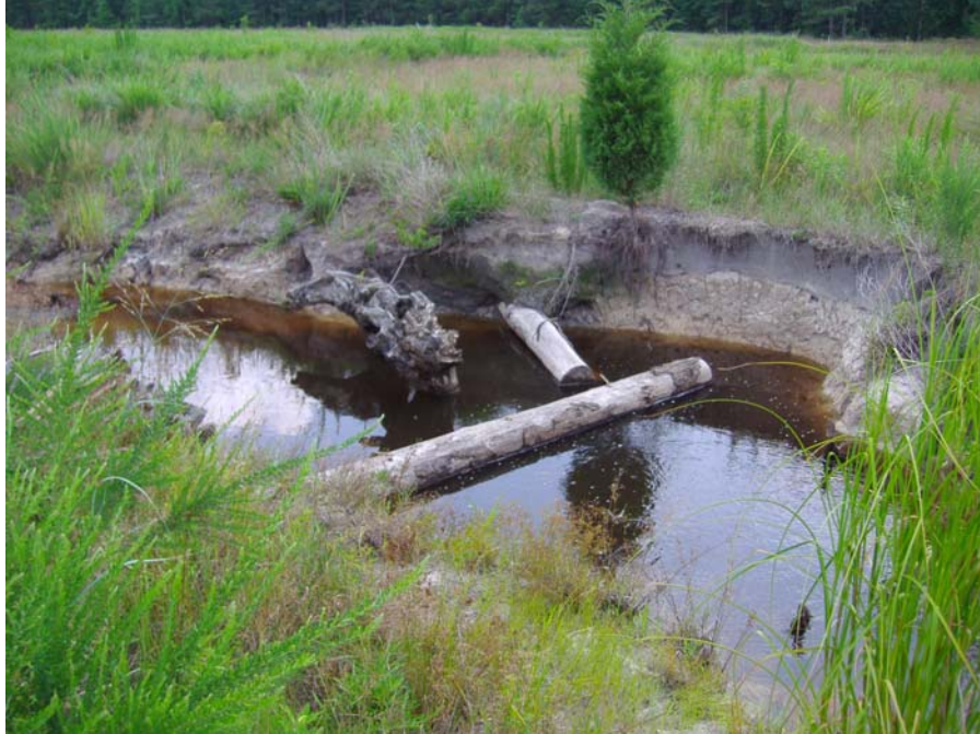
Photo 3. Failed log cross-vane structure downstream of the headcut. The logs were not notched together, allowing the arms to separate from the cross log. (7/4/07)
