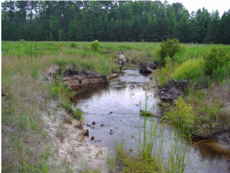
Photo 4. Typical example of a structure that has been washed away and resultant bank erosion (7/4/07)
