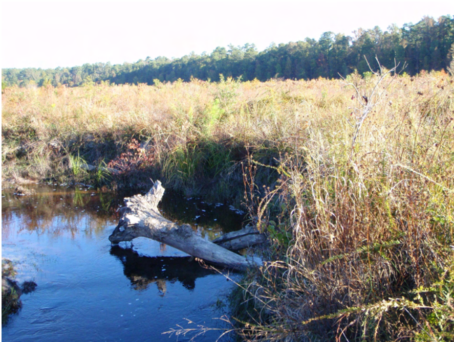
Photo 2. Looking upstream at failed bank and structure, near headcut at Sta. 33+00 (10/23/08).
