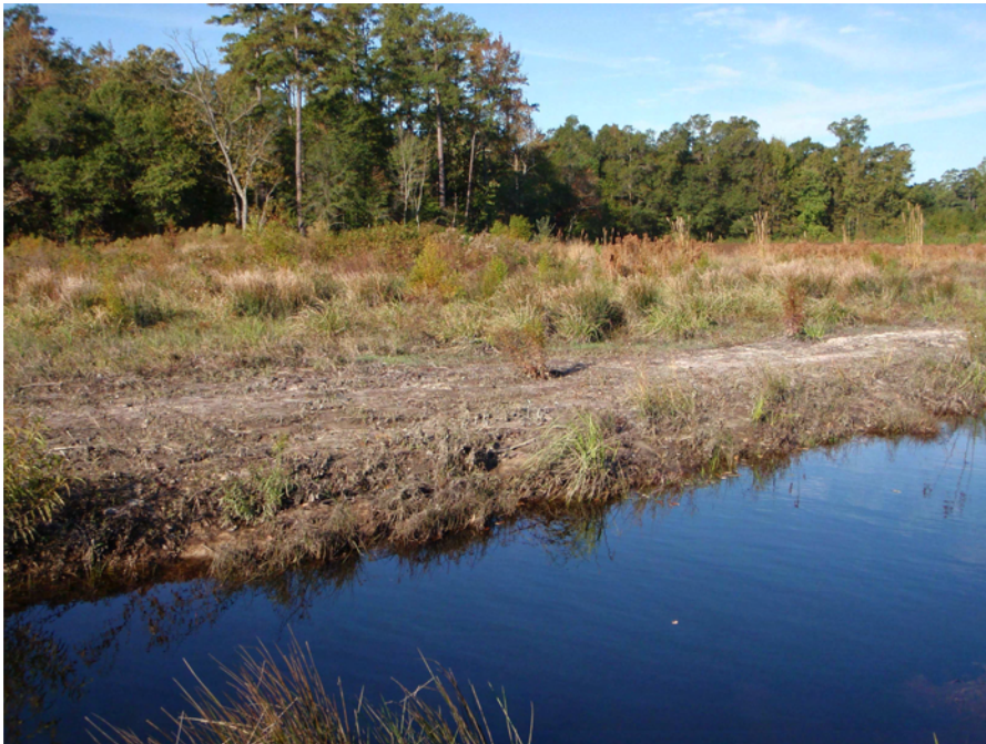
Photo 4. Bare floodplain and minor bank scour (10/23/2008).
