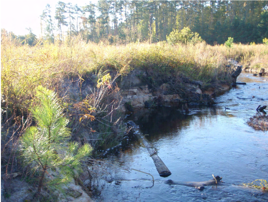
Photo 1. Looking downstream at a severely eroded bank and failed structure (10/23/08).
