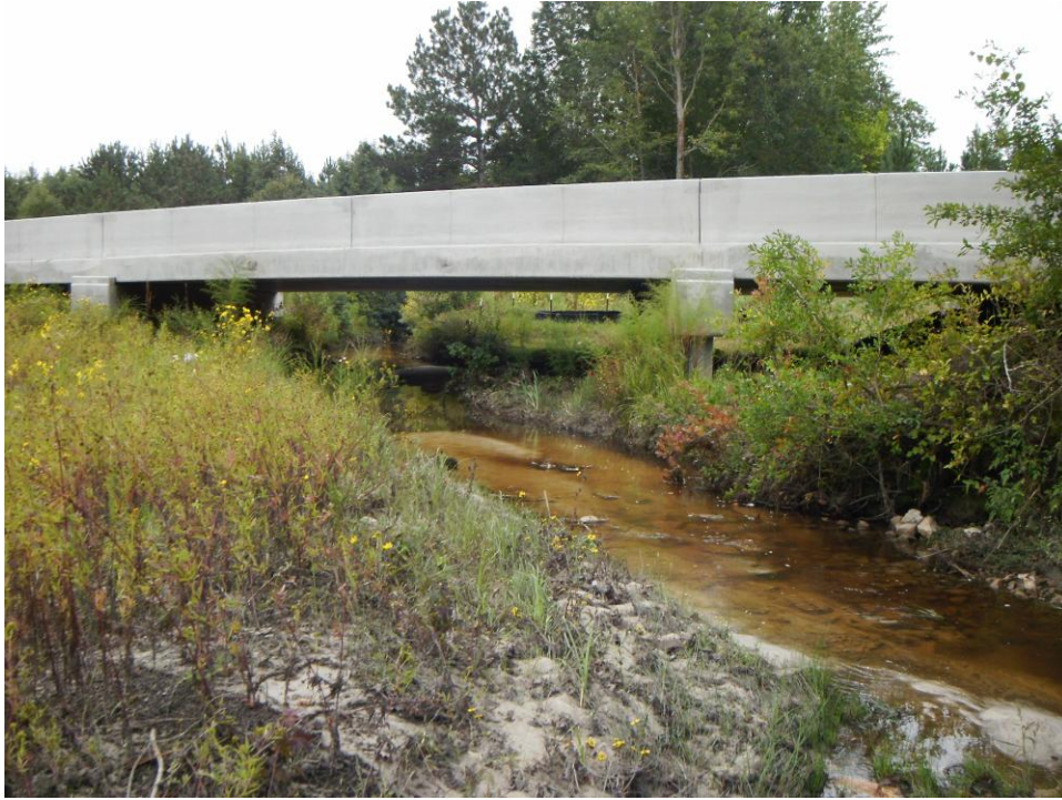
Photo 1 – Evidence of bankfull overflow near Station 42+00 – sediment on floodplain (9/21/11)
