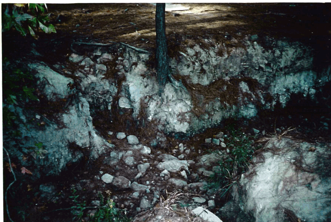
Unnamed Tributary to Bushy Branch eroding banks. Note lack of vegetation due to foot traffic.
