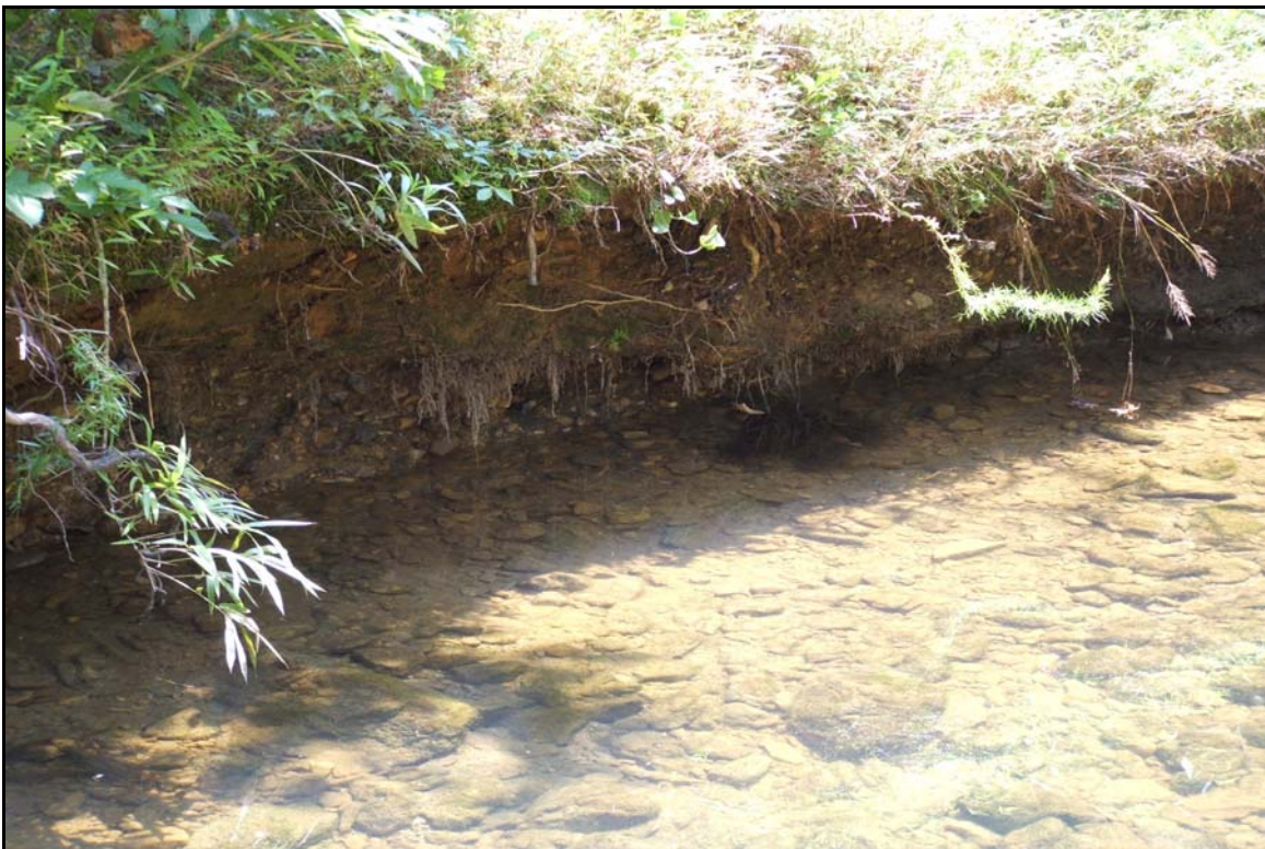
SP2 – Bank erosion. Photo taken near station 18+00. 10/27/05 - MY 01
