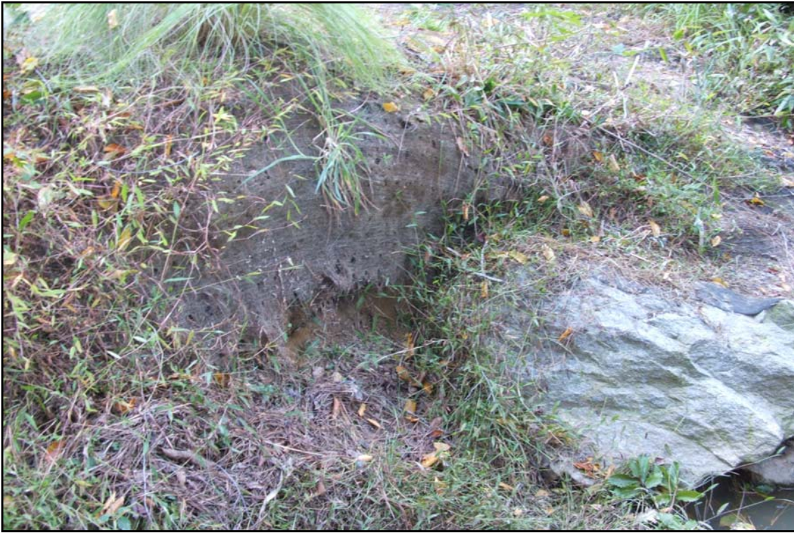
SP5 – Unstable, steep bank on UT to Bushy Creek, near confluence with Busy Creek. Photo taken near station 03+30. 10/27/05 - MY 01
