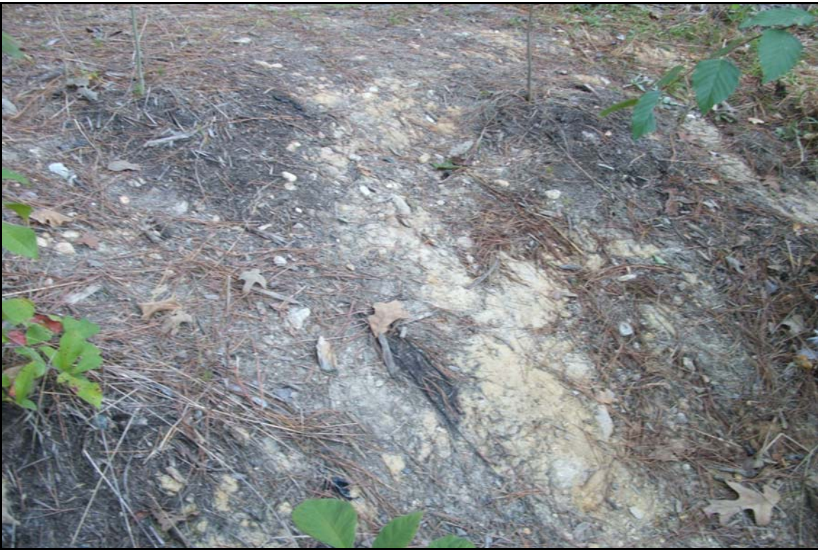
VP8 – Breakdown of geogrid stabilization, with bare subsoil exposed on stream bank. Photo taken near station 00+30. 10/27/05 - MY 01
