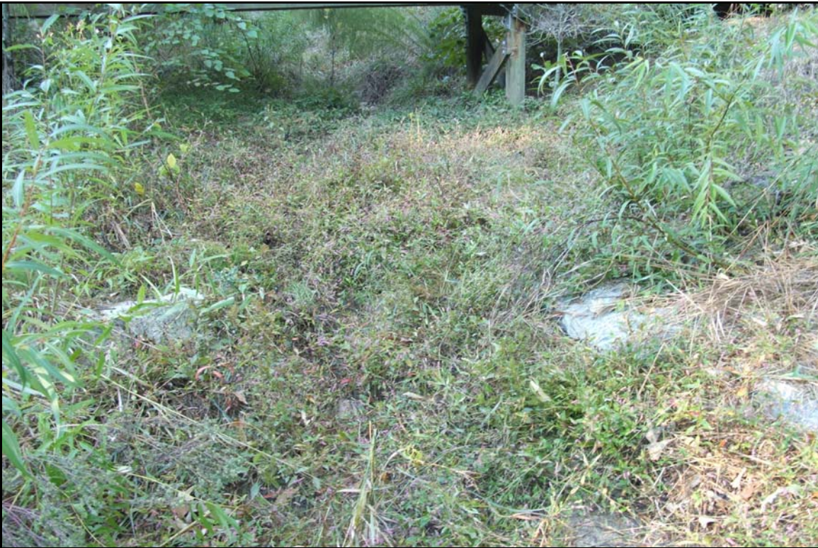
SP4 – Bed aggradation and weedy growth in channel. Photo taken near station 02+00. 10/27/05 - MY 01
