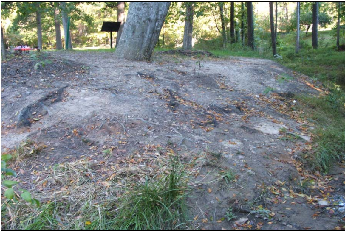
VP1 – Bare terrace occurs near the confluence of Bushy Branch and the UT. Photo taken near station 12+00. 10/27/05 - MY 01
