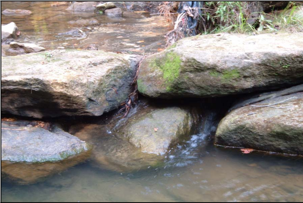
SP3 – Piping through boulders in cross vane. Photo taken near station 16+00. 10/5/06 - MY 02
