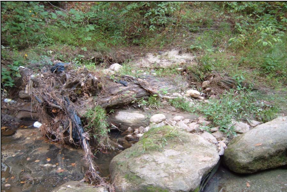
SP4 – Scour behind root wads. Photo taken near station 16+00. 10/5/06 - MY 02
