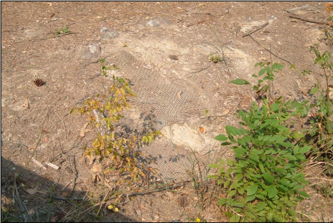
VP5 – Breakdown of coir matting, with bare subsoil exposed on stream bank. Photo taken near station 03+40. 10/5/06 - MY 02
