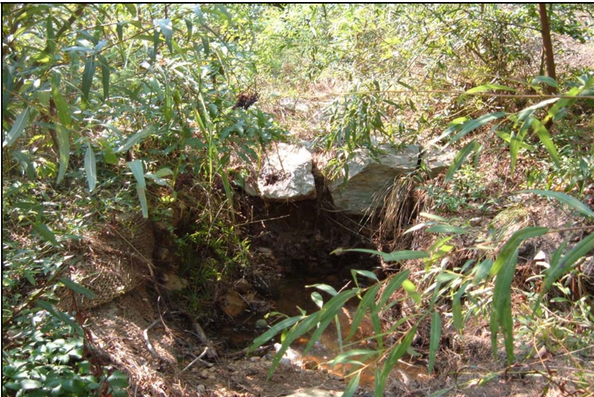
SP6 – Bed degrading on downstream side of rock sill. Photo taken near station 02+25. 10/5/06 - MY 02
