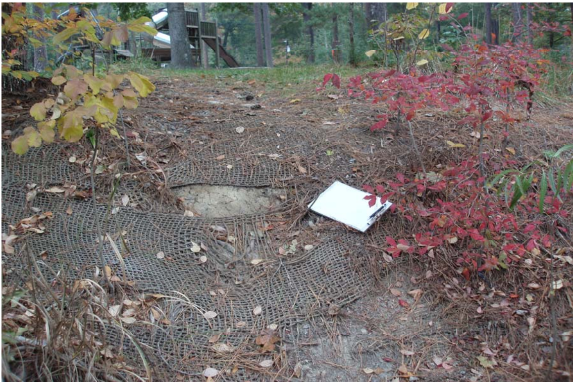
VP4 - Breakdown of coir matting with bare subsoil exposed on stream bank. Photo taken near Station 02+00. 11/12/07 - MY 03
