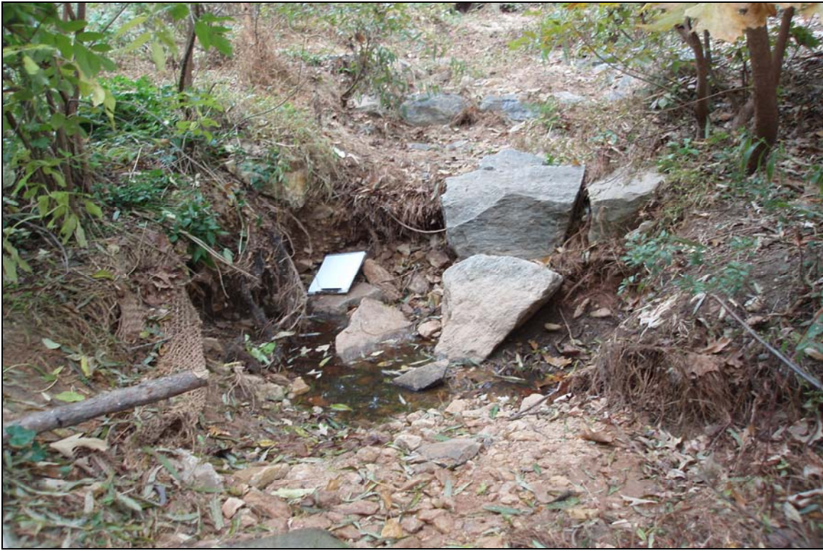
SP5 - Head stones of cross vane fallen into pool with headcutting. Photo taken near Station 2+20. 11/12/07 - MY 03
