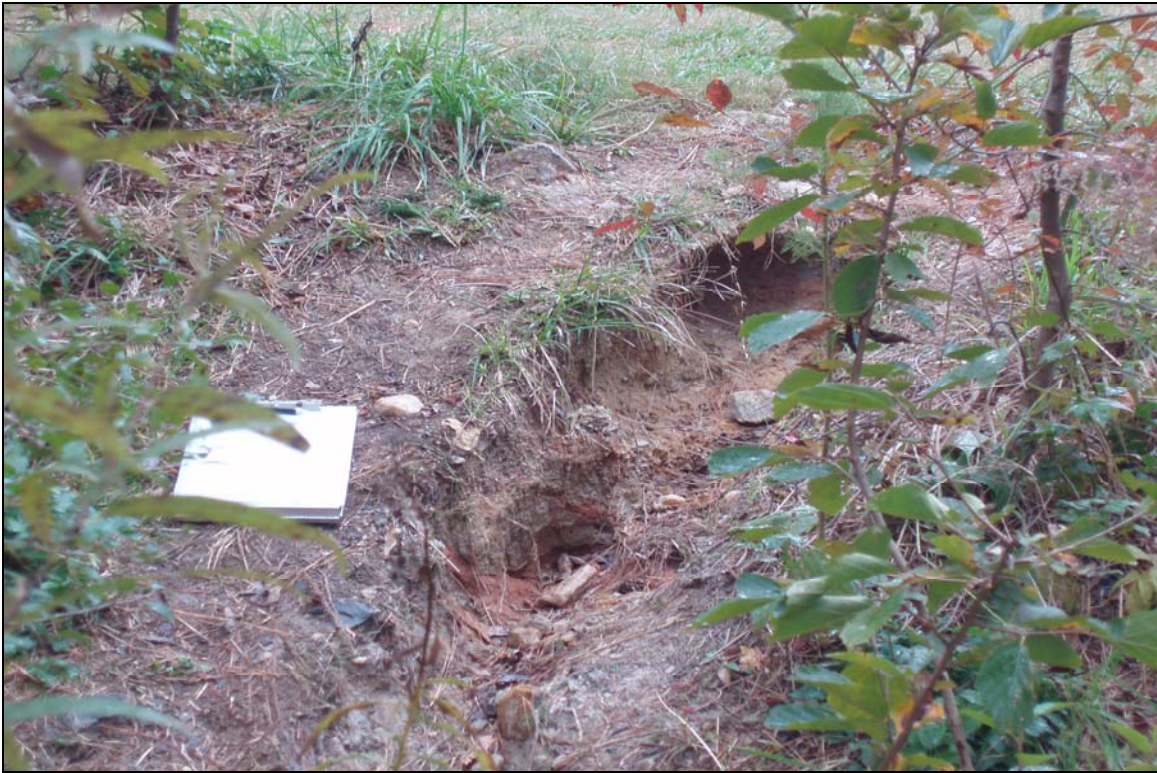
VP5 - Erosion from path worn into stream bank from pedestrian access to the stream. Photo taken near Station 01+00. 11/12/07 - MY 03
