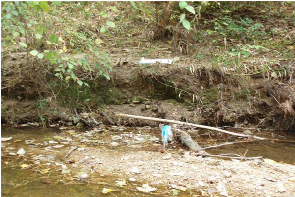
SP1 - Bank erosion. Photo taken near Station 17+80 on left bank. 10/28/08 - MY 04
