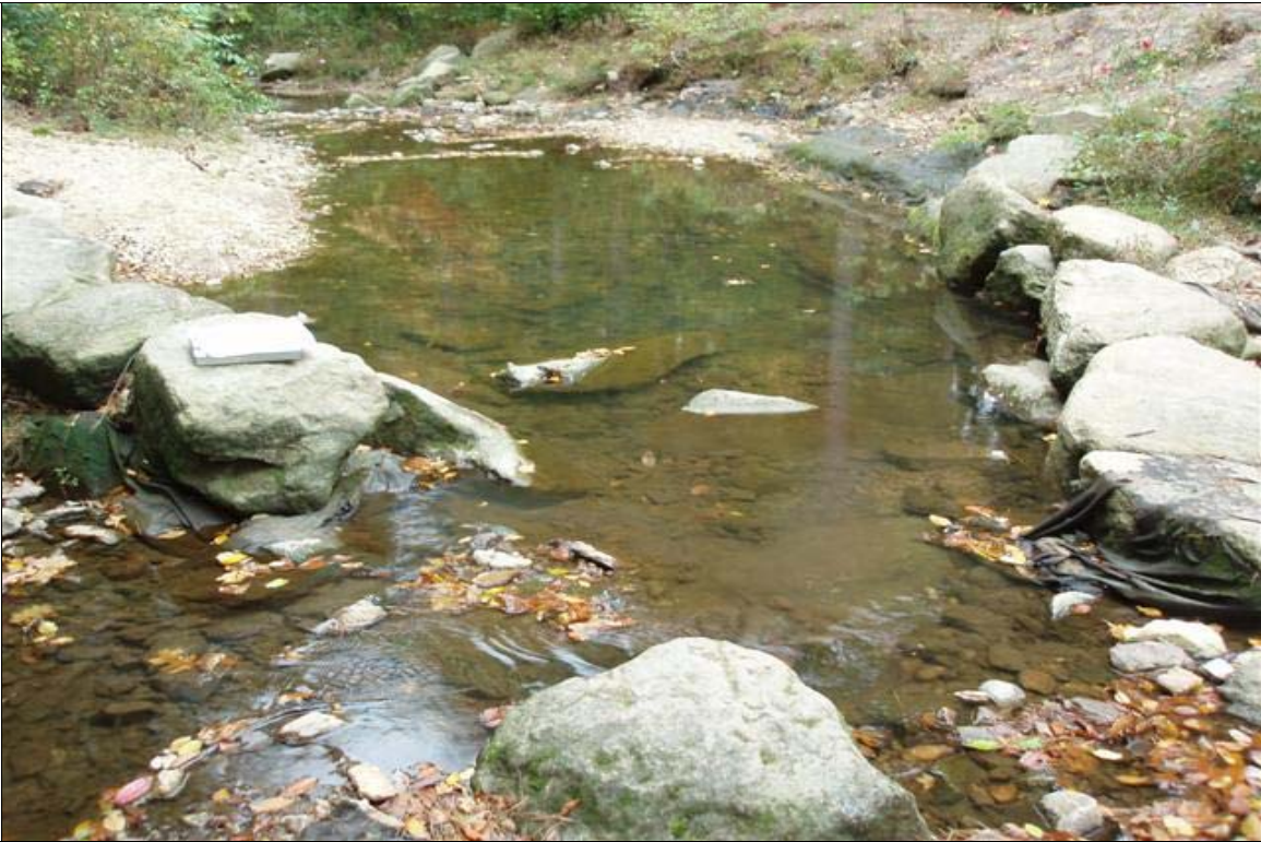
SP3 - Failed cross vane in main stem. Photo taken near Station 12+60. 10/28/08 - MY 04
