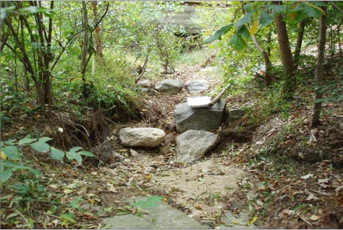
SP5 - Header stones of cross vane that have fallen into the pool; the stream is headcutting up from this point. Photo taken near Station 02+20. 10/28/08 - MY 04
