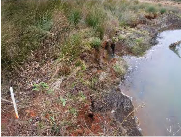
Bull Creek R2 Left Bank Scour/ Eroded at PP4 – looking downstream (12/30/2020)
