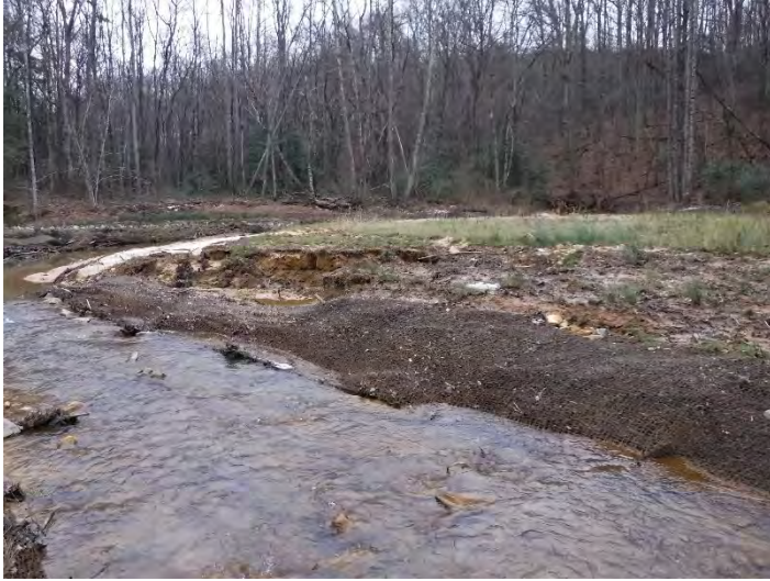
Bull Creek R3 Right Bank Scour at Station 165+50 – looking downstream (12/30/2020)
