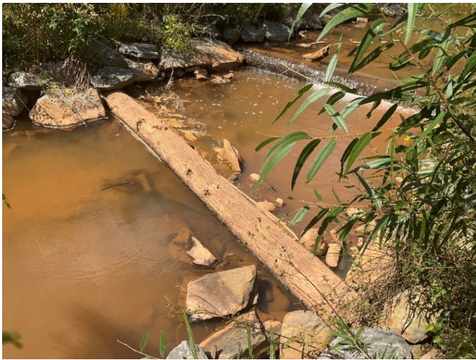
Bull Creek Reach 3: log roller riffle at station 164+00 with piping under one of the structure's logs – looking upstream (09/19/2022)
