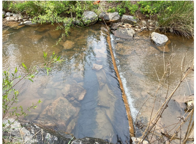
Bull Creek Reach 3: Filter Fabric added and secured to log roller at station 164+00, water is no longer piping (04/25/23)
