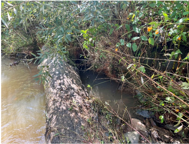
Bull Creek Reach 2: J-hook structure at station 115+30 with piping starting to occur from bank erosion (09/13/2023)
