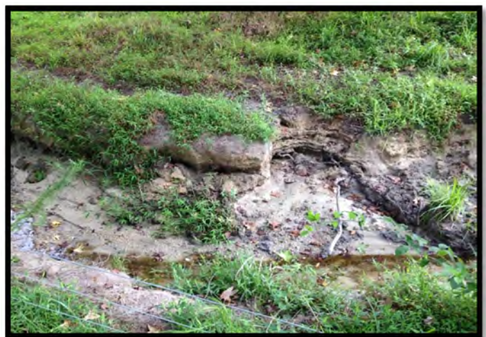
Looking at right bank erosion and sediment deposition along R2. Note the lack of deep rooted vegetation.
