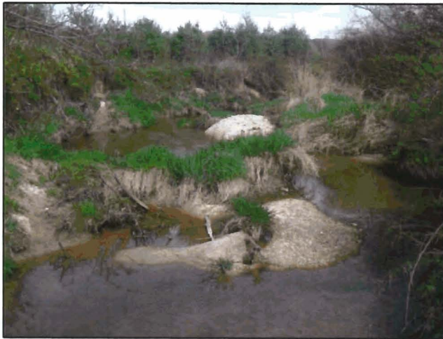
1. Main Channel Bank Erosion 7.3.2007
