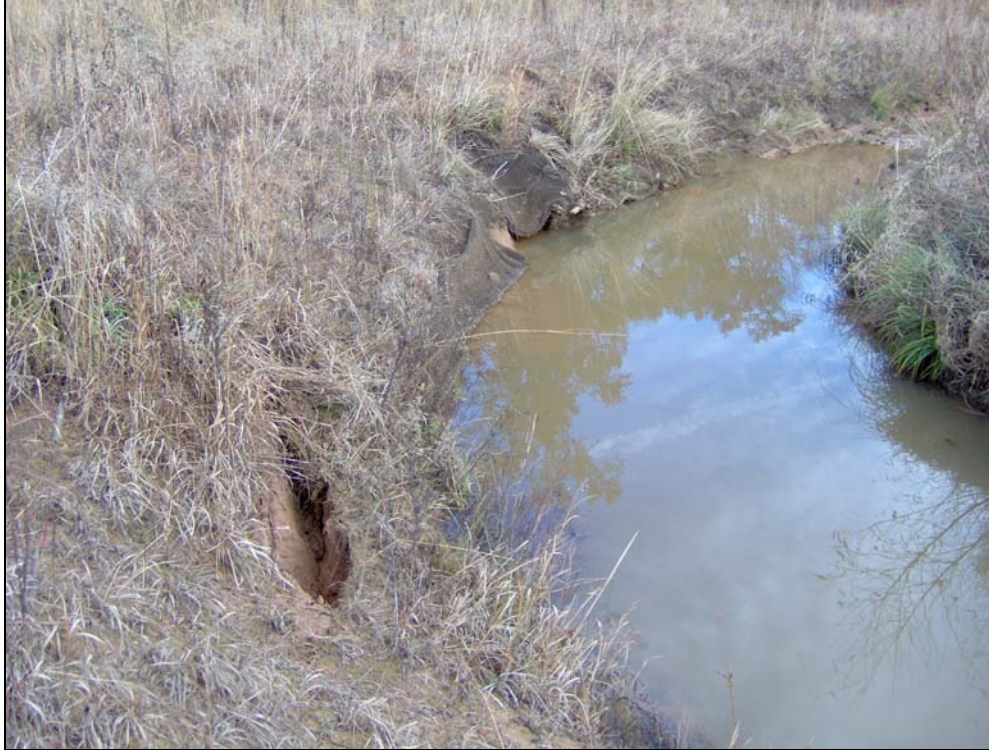
Representative toe scour on outside of bend, Lick Creek STA 40+50 11/27/07 Photo No. 24
