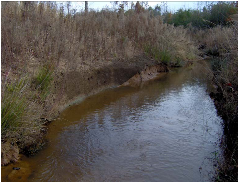
Toe Scour on Lick Creek, STA 23+00 11/27/07 Photo No. 18
