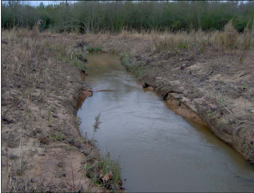
Toe Scour on Lick Creek, STA 23+00 12/03/06 Photo No. 17
