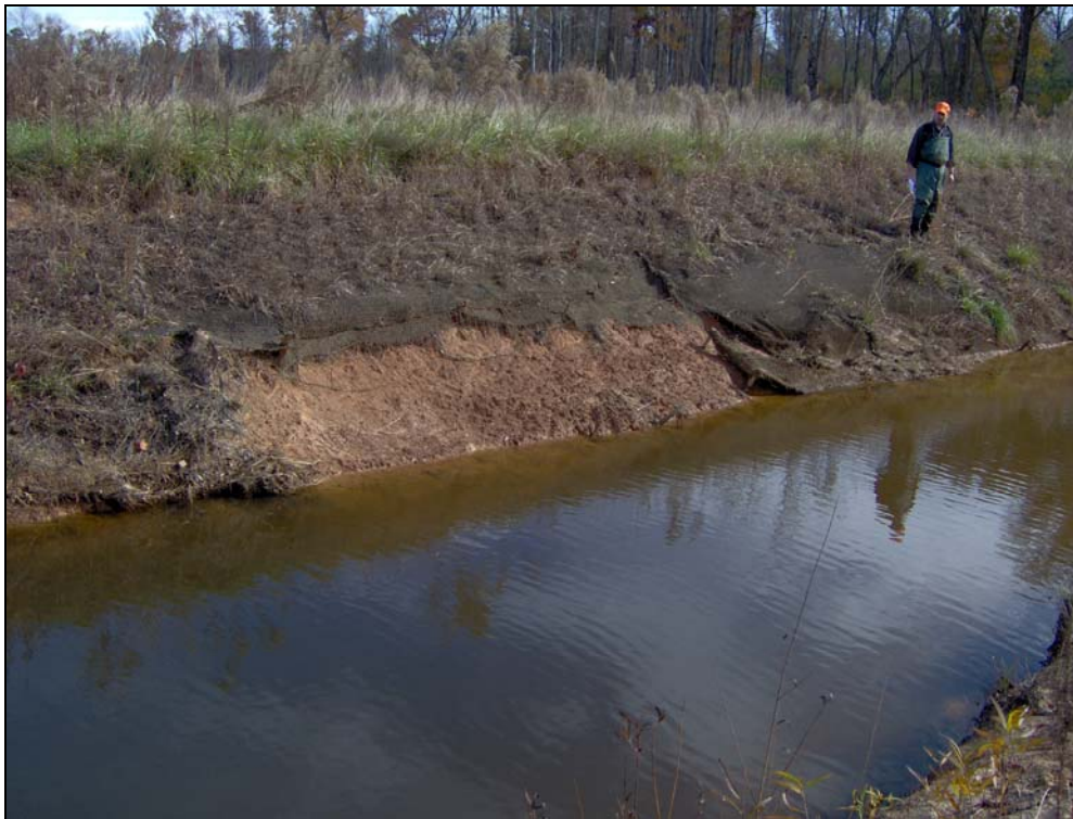
Loss of Matting, Lick Creek STA 37+50, 11/27/07 Photo No. 25
