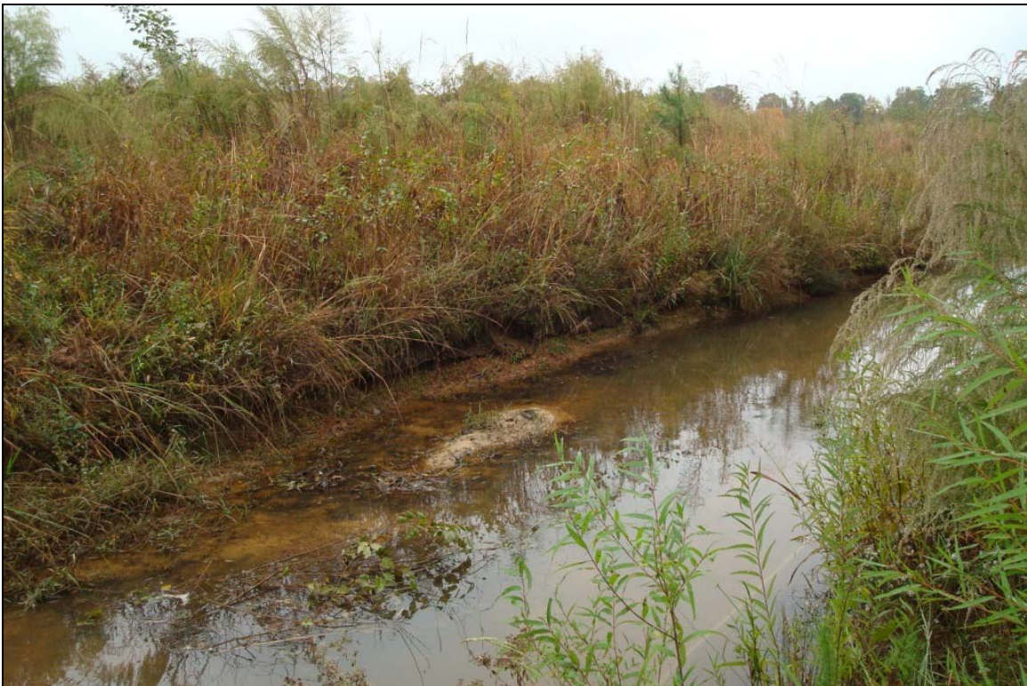
Toe Scour at Lick Creek, Sta 40+25
