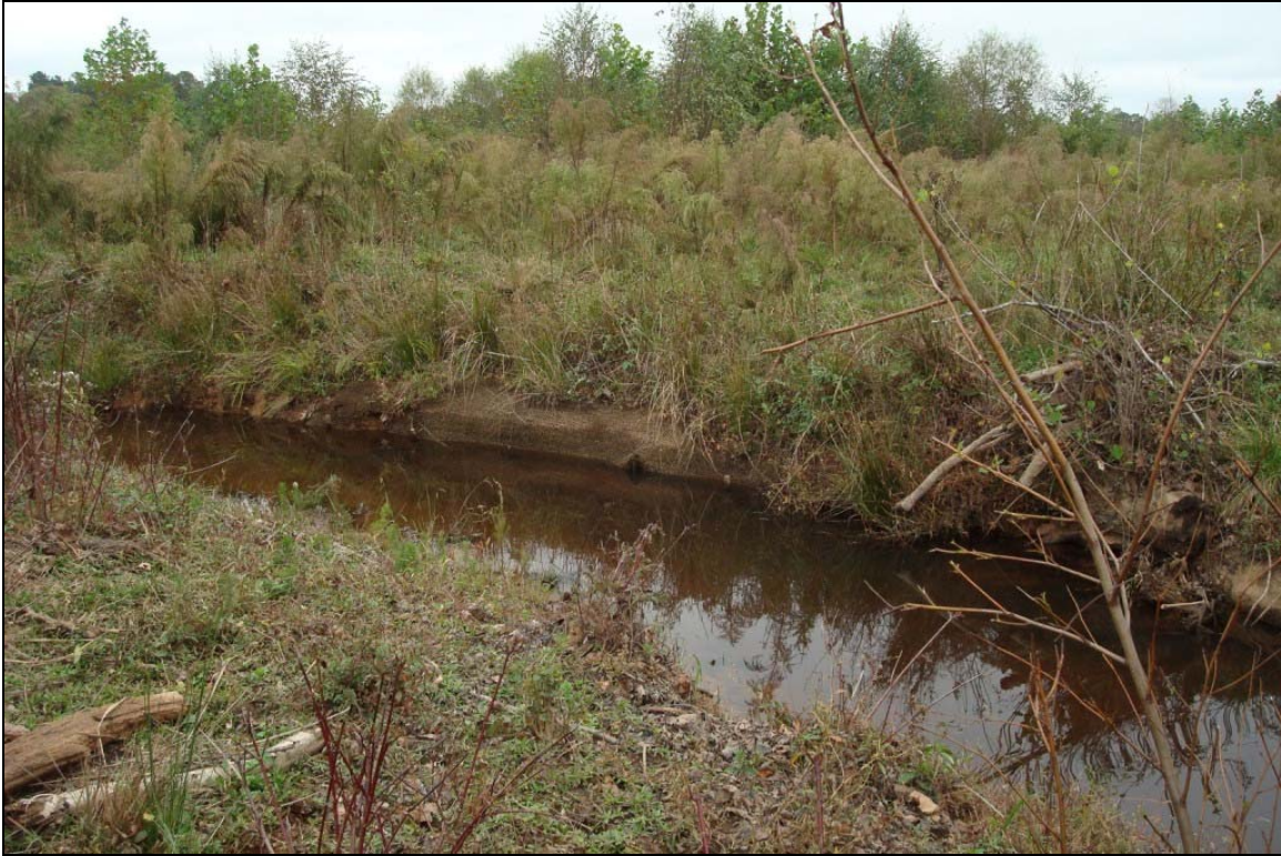
Bank Erosion at Wallace Branch, Sta 13+90
