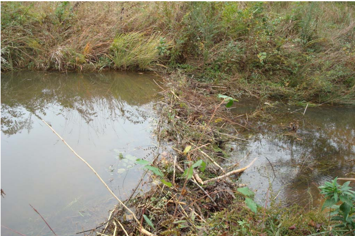
Beaver Dam on Lick Creek, Sta 61+00
