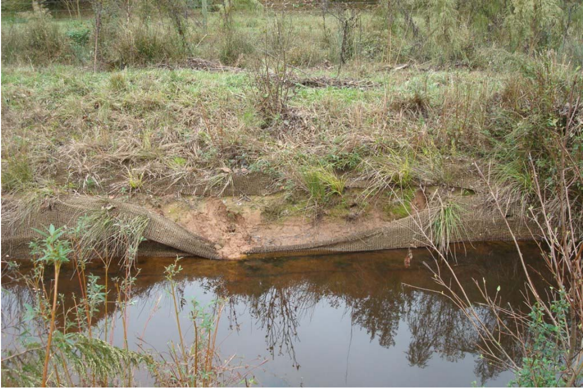
Banks Impacted by Cattle on Wallace Branch, Sta 12+30 Photo No. 23
