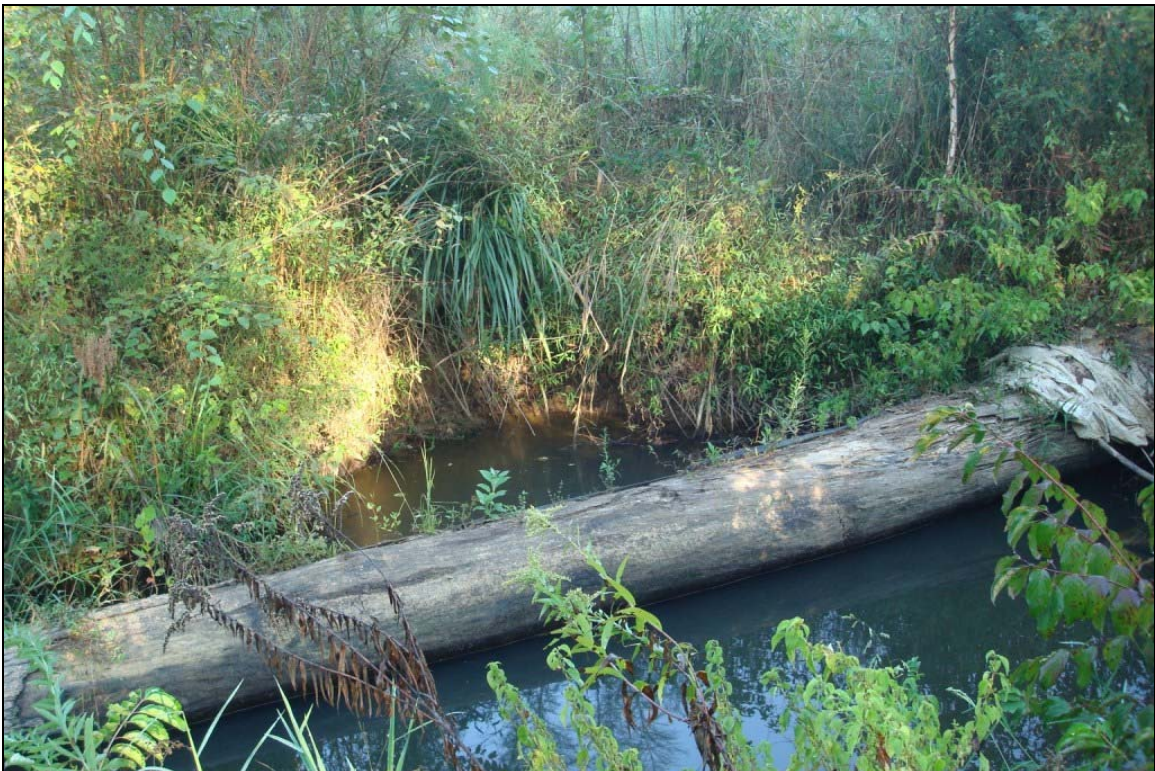
Scoured Log Vane Arm, Lick Creek, Sta 10+80 Photo No. 18
