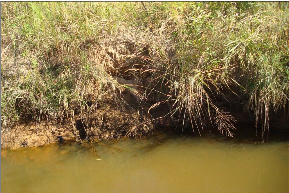
Minor Toe Scour, Lick Creek, Sta 50+30
