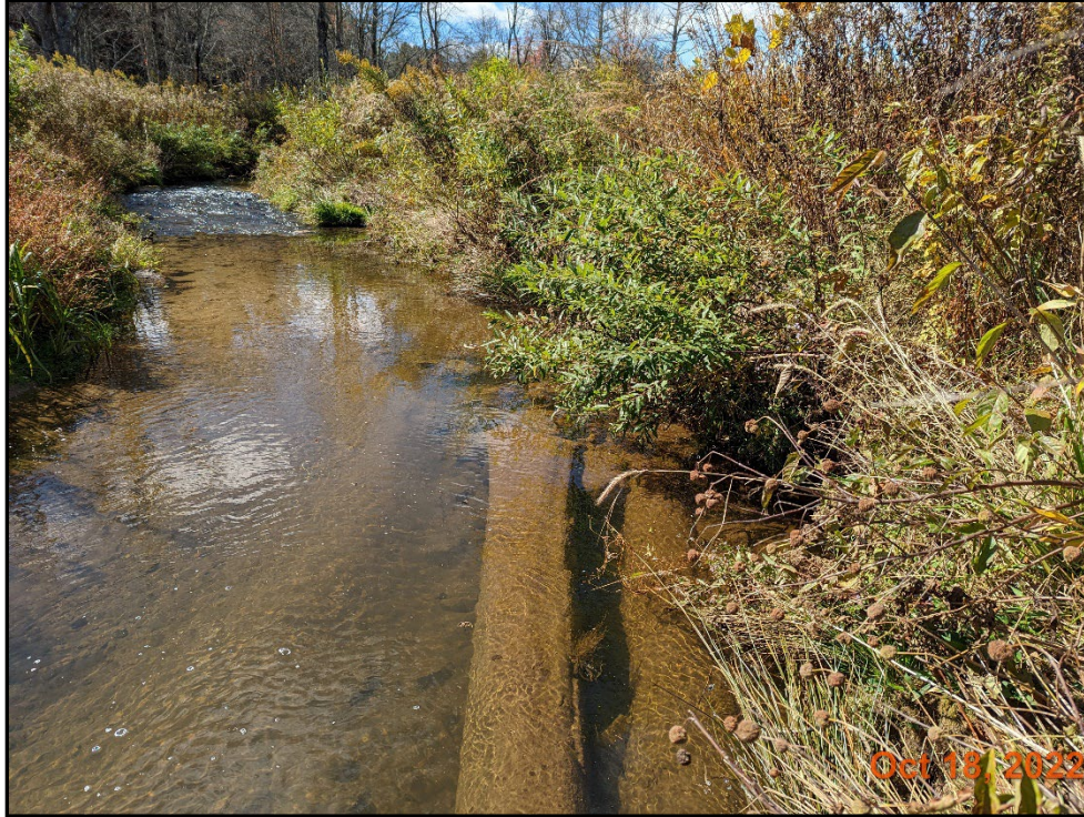
Little Pine Creek II Reach 2A – Exposed structure Station 113+30
