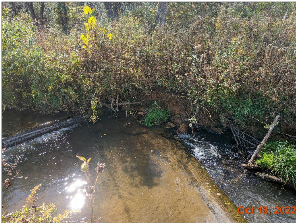
Little Pine Creek II Reach 2B –Bank Erosion Station 121+75 facing left descending bank
