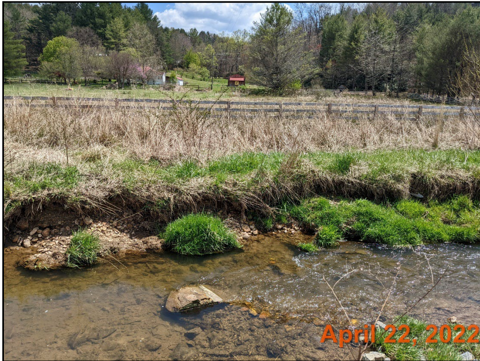
Little Pine Creek II Reach 1– Bank Erosion Station 110+20
