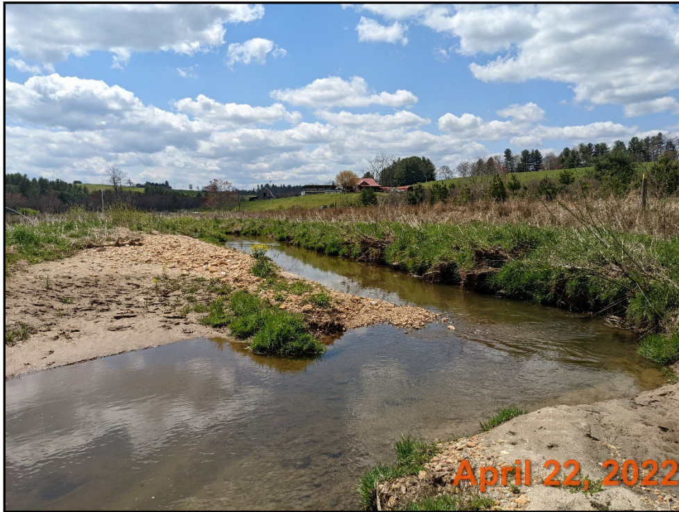
Little Pine Creek II Reach 1– Bank Erosion Station 100+10
