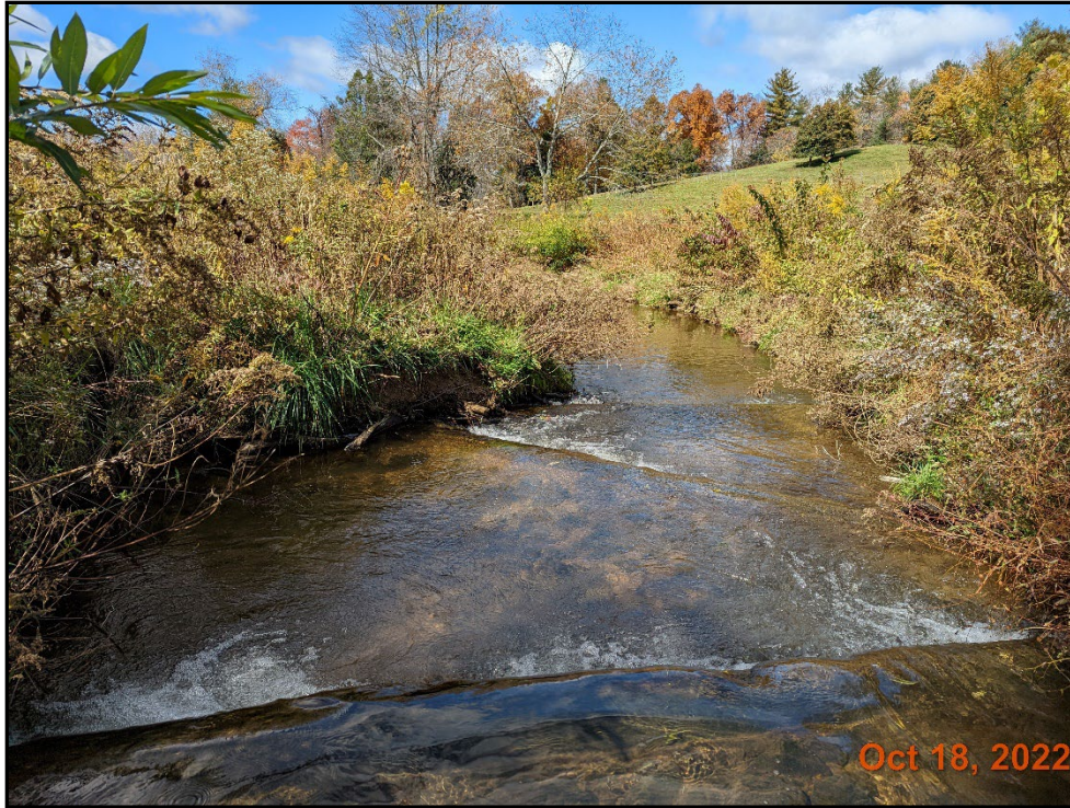
Little Pine Creek II Reach 2A – Bank Erosion 118+00, facing downstream
