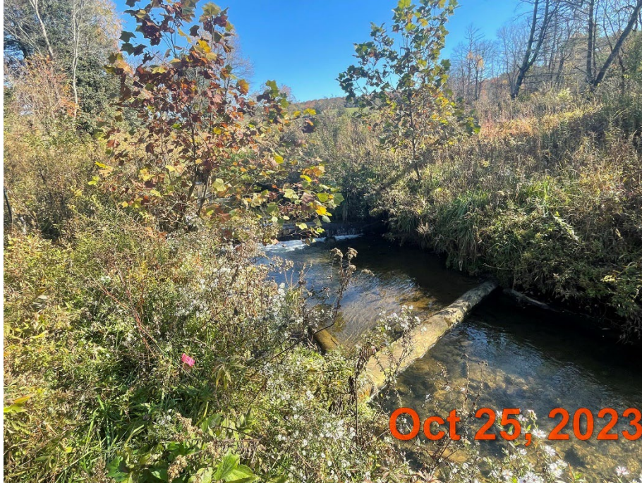
Example undercut bank and toe structure exposure along Reach 2B.
