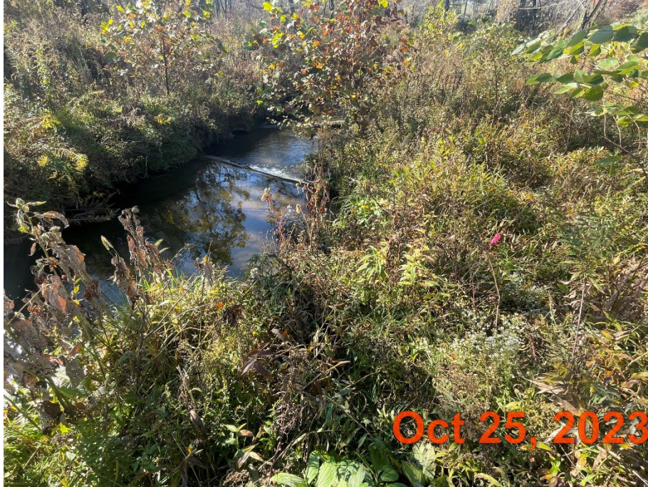
Example slump bank along Reach 2B.
