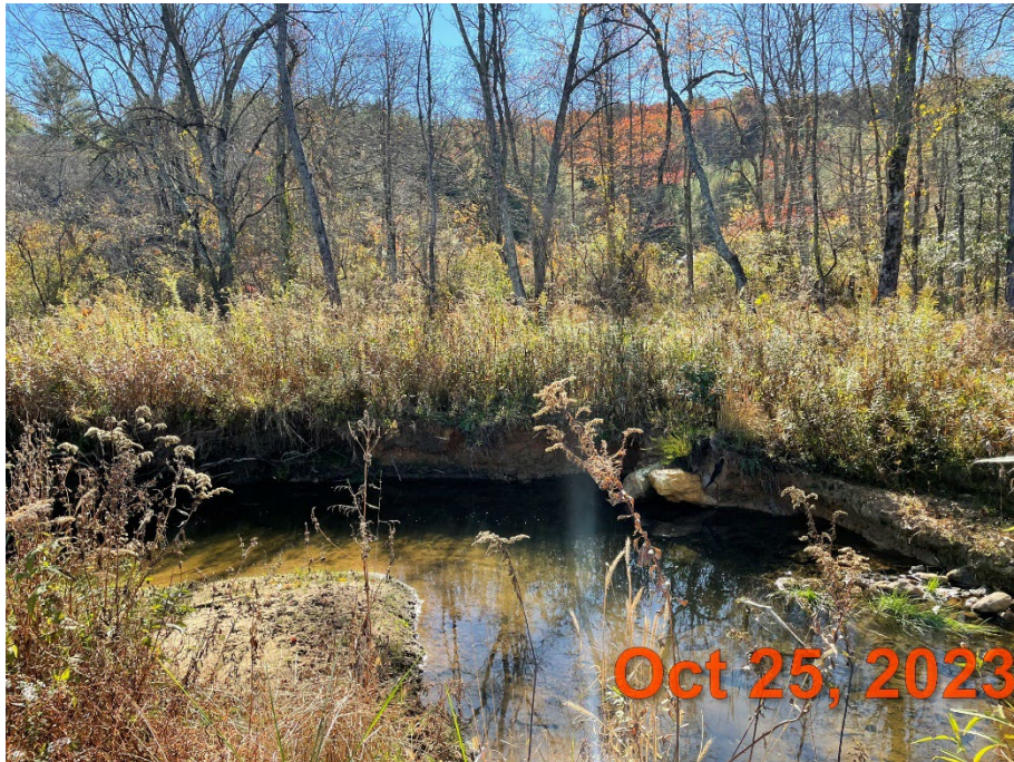
Example undercutting along Reach 2A.
