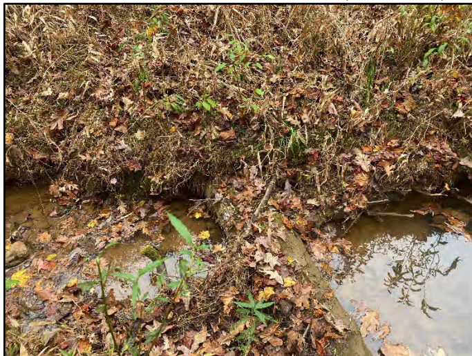
Failing Log Sill BS1-C / Stream Problem Area #3 (10/31/2023)
