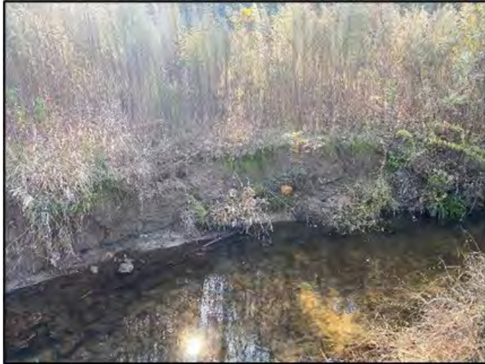
Right Bank Erosion & Brush Toe Failure on MC1-C / Stream Problem Area #1 (10/31/2023)
