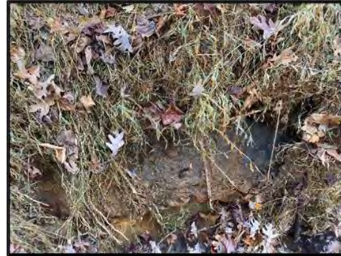
Right Bank Erosion BS1-C / Stream Problem Area #2 (11/7/2023)
