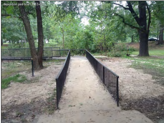
Alluvial deposition from flooding on the pedestrian bridge at XS1.
