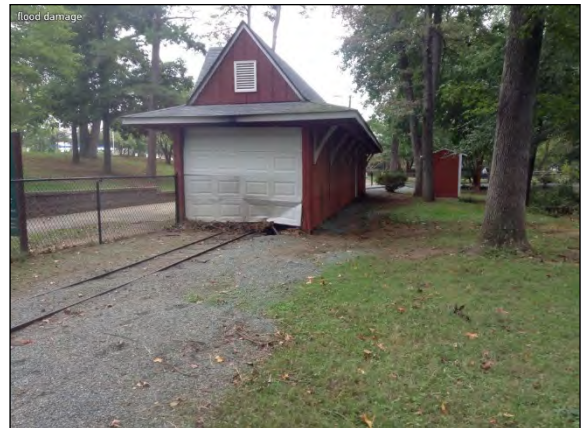
Damage to train garage from debris in flash flood event.
