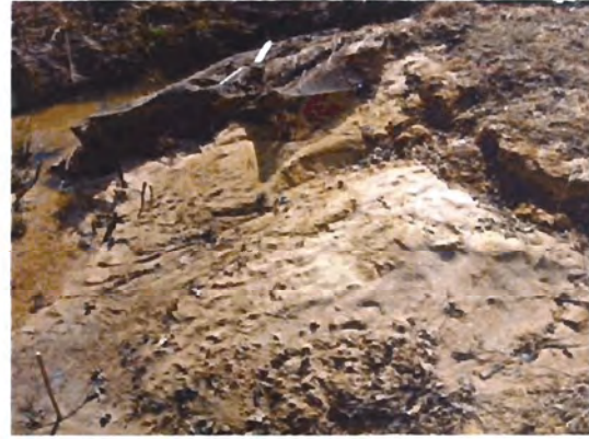
VPA 2. Eroded banks from lack of vegetation.
