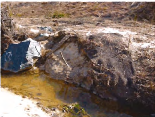
VPA 6. Live stakes not establishing allowing for eroded bank on left bank.
