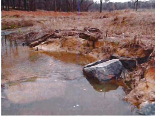
SPA. 22. Right bank scour around structure. Sta. 36+14.
