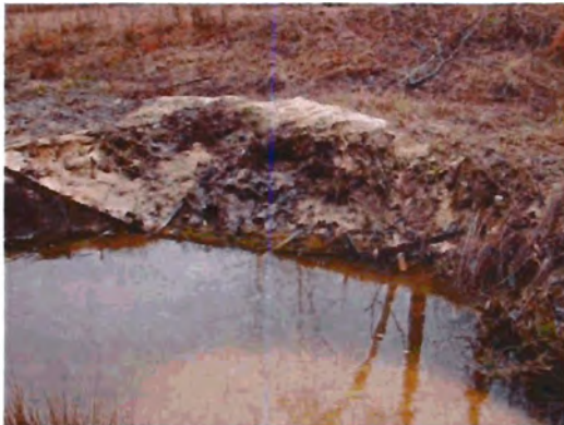
SPA 11. Coir matting dislodged. Sta. 21+91.
