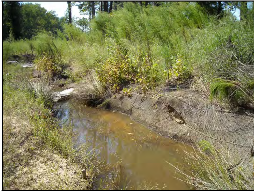
VPA 24. Left descending bank has bare coir matting and eroding banks.
