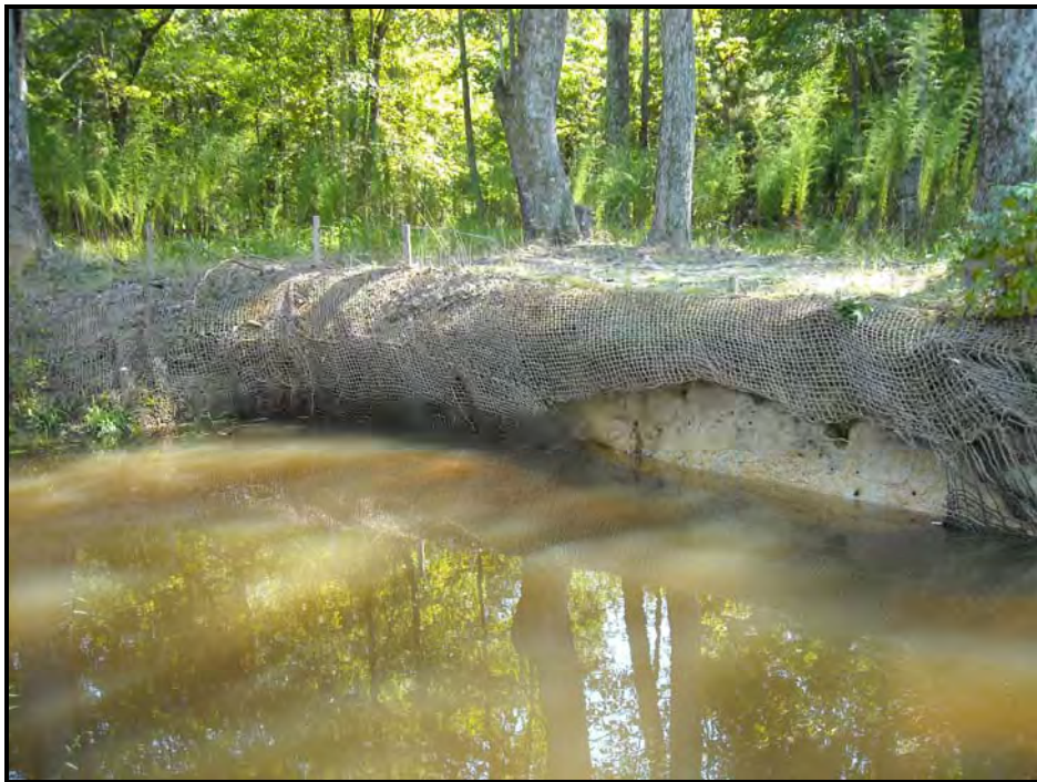
VPA 21. Left descending bank is eroding and is has bare coir matting.
