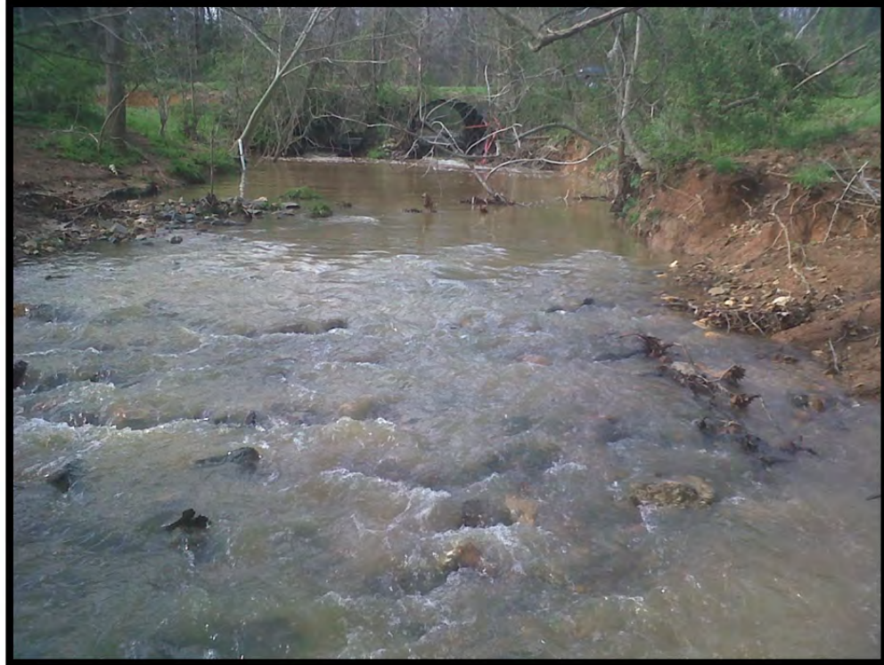
UT 7 – The culverts under Old Mine Road are the upstream limit of the restoration reach. (3/29/2010)
