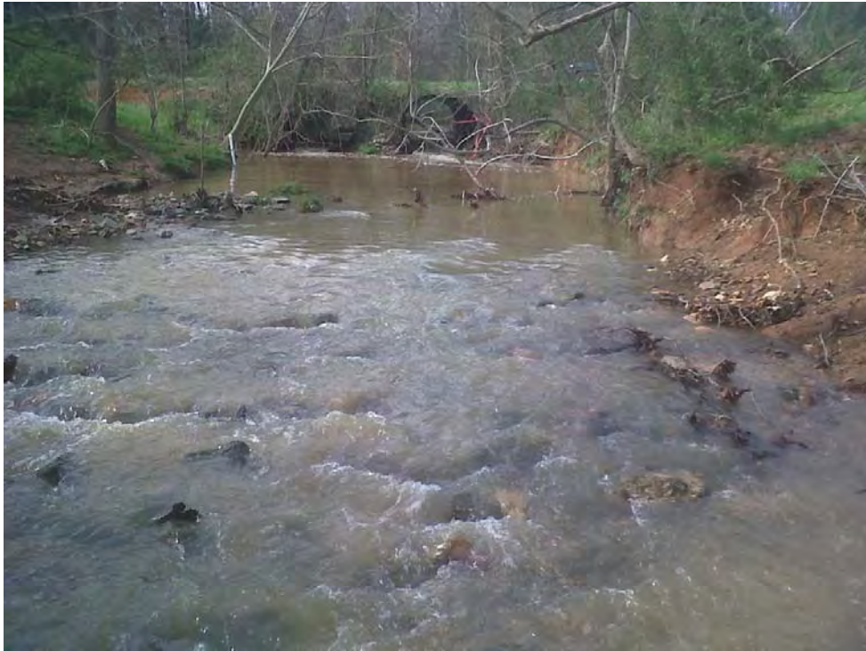
Photo 19: UT 7. View looking upstream at upper limit – culverts under Old Mine Rd. (3/29/2010)
