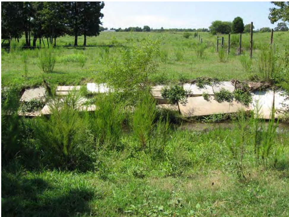
Photo 8: Reach 4. Concrete on rt. bank to be removed and dimension, pattern, & profile restored. (8/30/2010)
