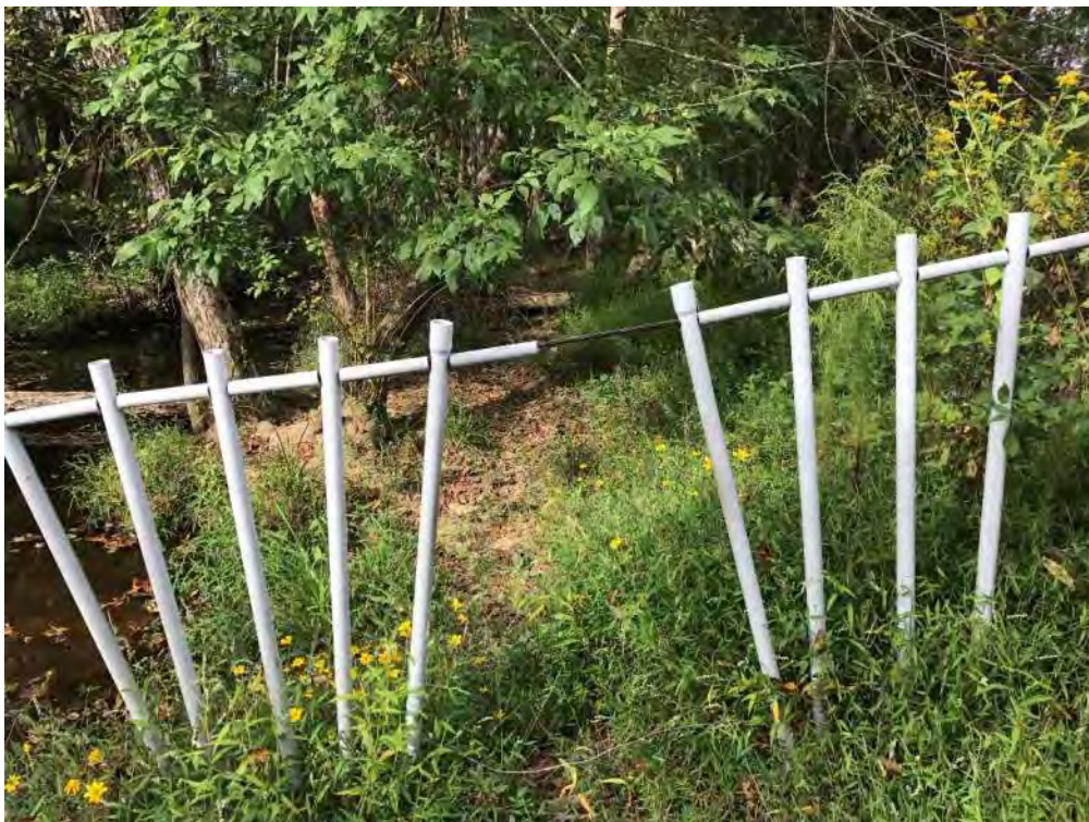
Cattle crossing opening in flood gate, with no electric power. Not being maintained by owners.
