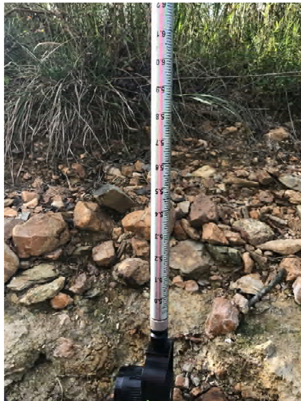
15 foot bank scour along the right Bank in restoration area of reach 4
