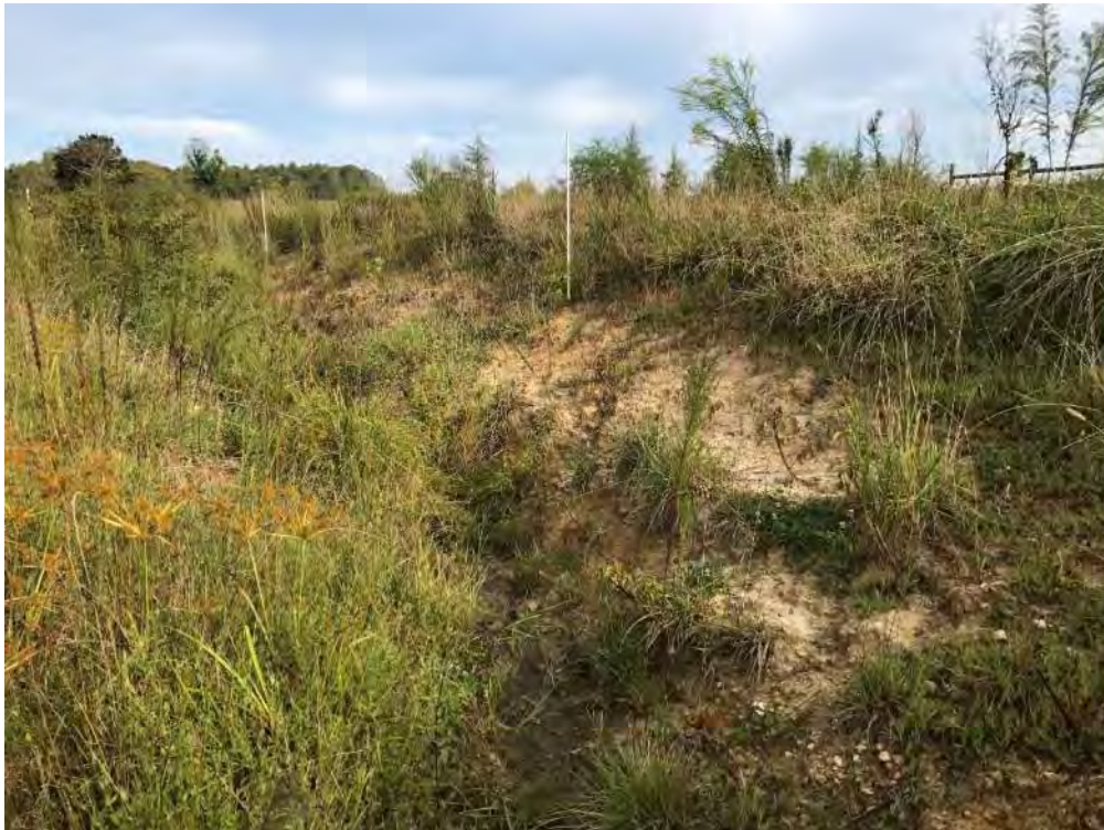
Poor vegetation along portion of left bank in UT3
