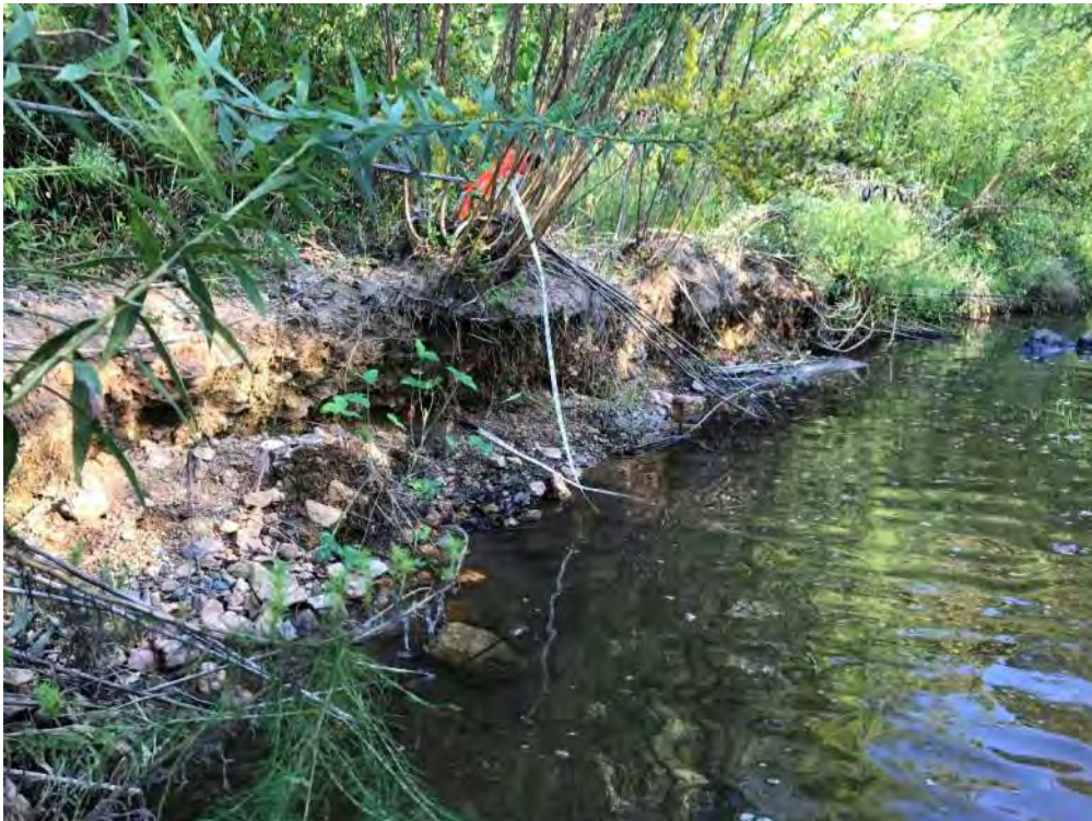
Undercut along the left interior channel bank in restoration area of reach 3
