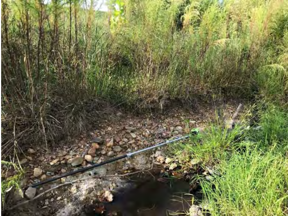
15 foot bank scour along the right bank in restoration area of reach 4
