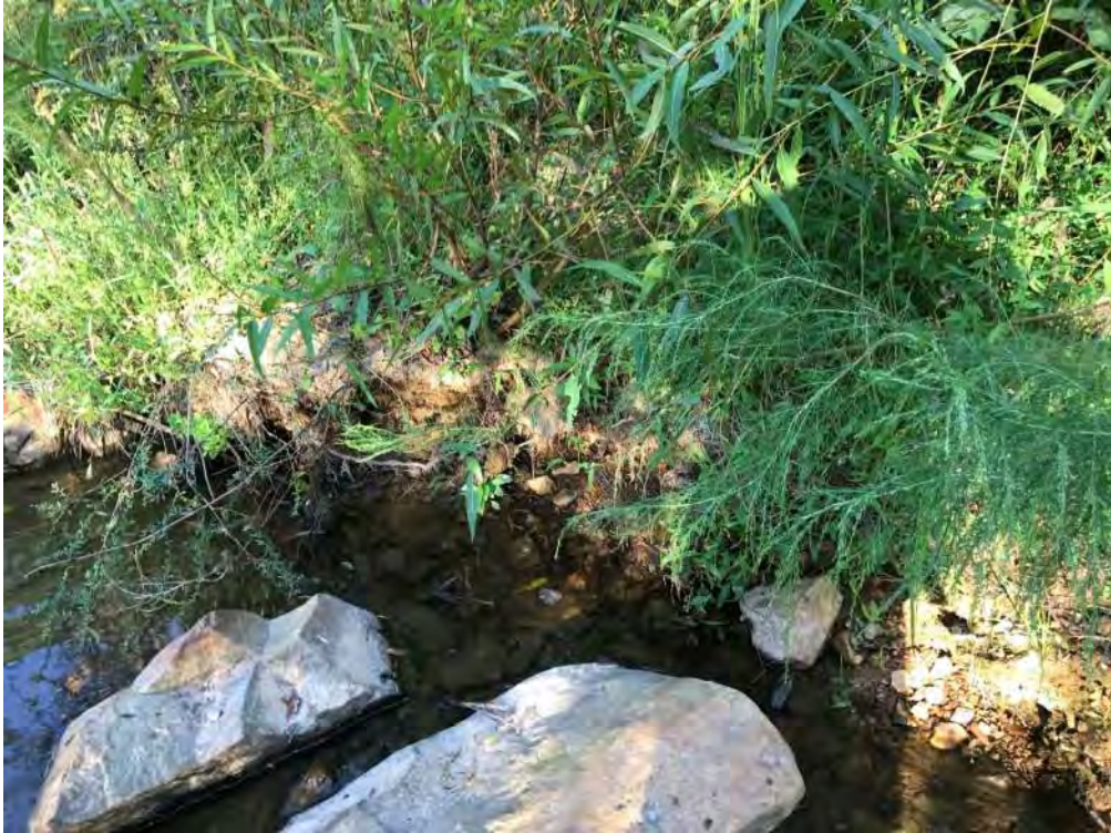
Undercut along the left interior channel bank in restoration area of reach 3
