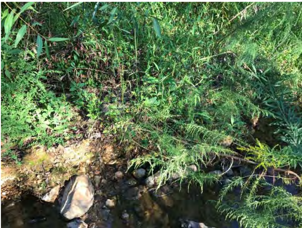
Undercut along the left interior channel bank in restoration area of reach 3
