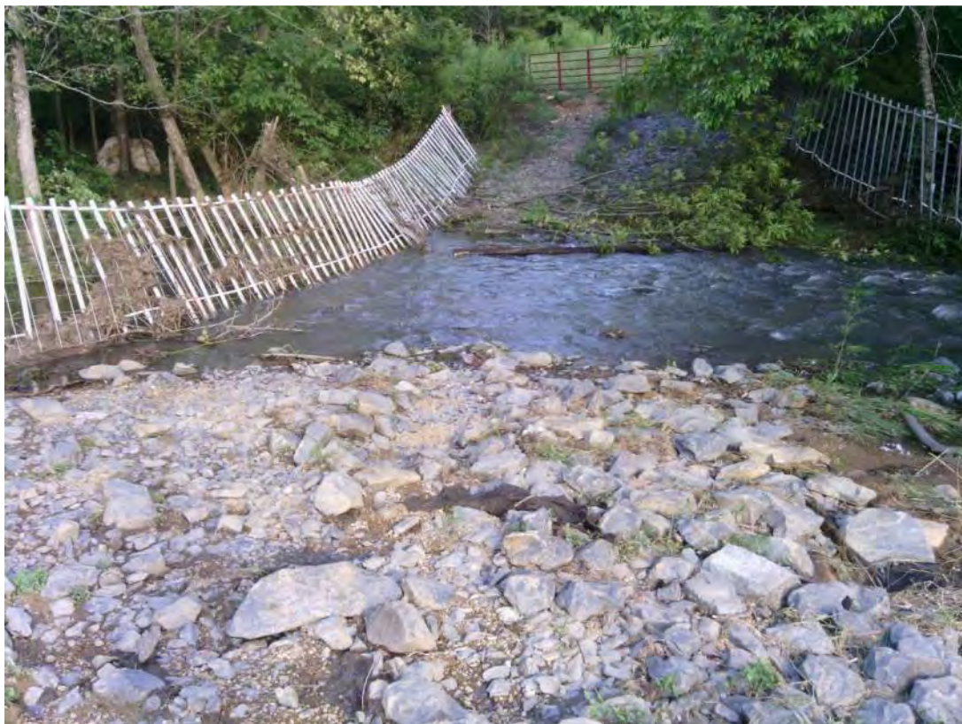
Blown out cattle crossing (Reach 5)
