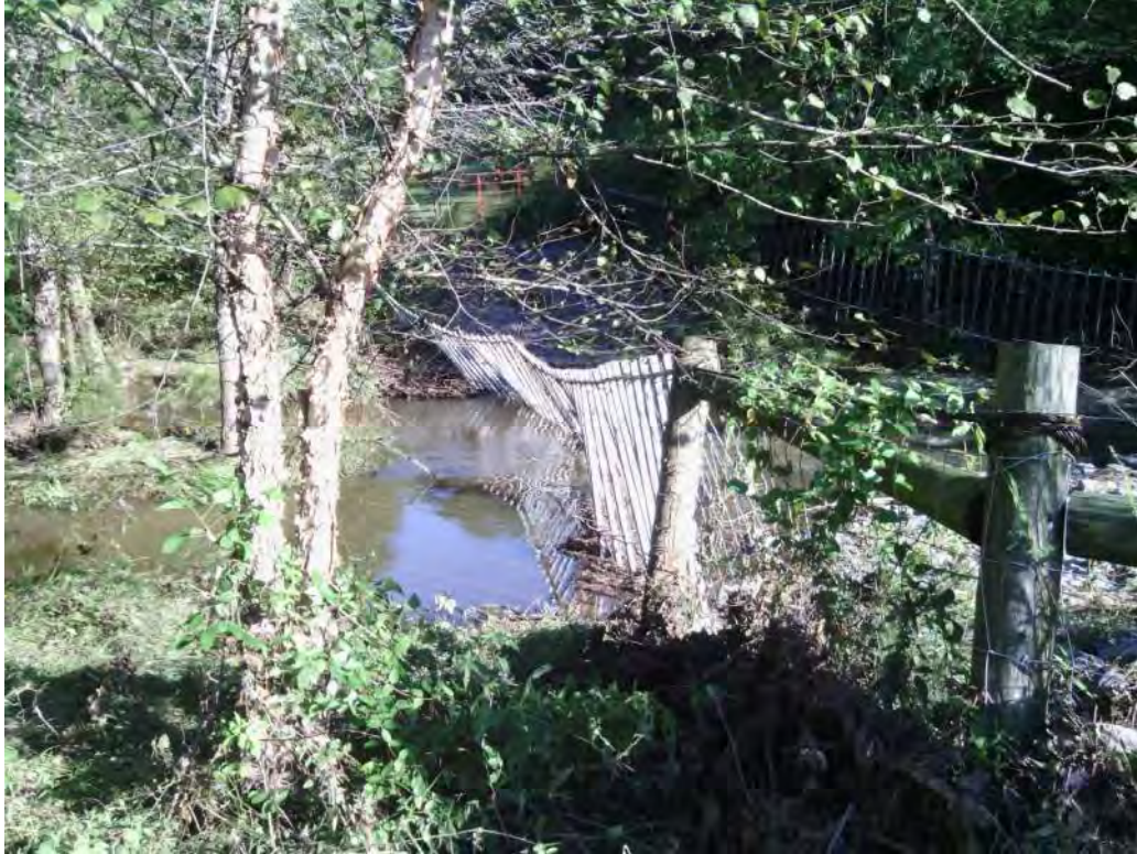
Blown out cattle crossing (Reach 5)
