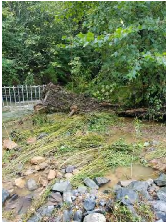
Wreck line at cattle crossing from Hurricane
