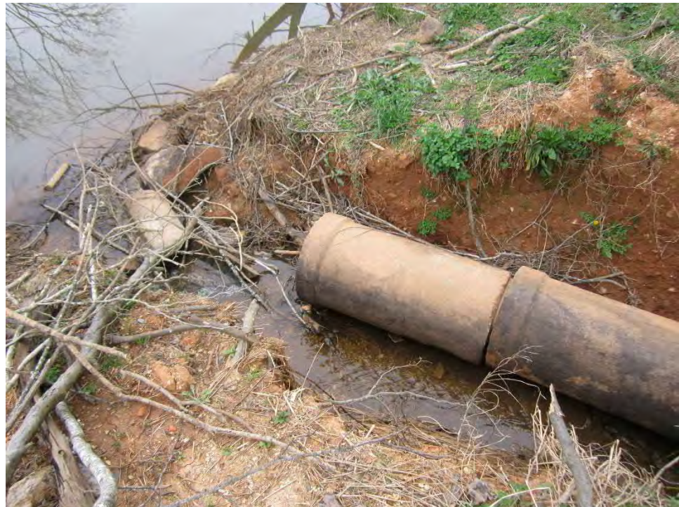
Dam blowout around existing concrete outlet pipe (US end of UT2)
