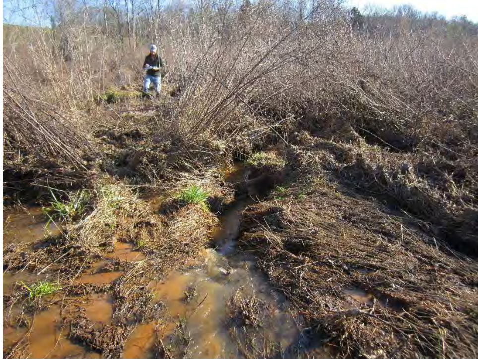
Small headcut in UT2 near Station 16+85 (January 2020)
