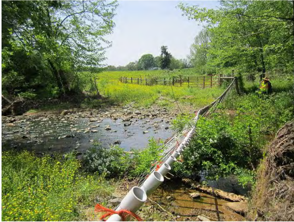
Blown out cattle crossing (Reach 5)
