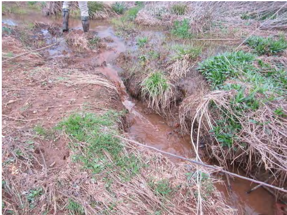
Headcut in UT2 near Station 16+95 (March 2020)
