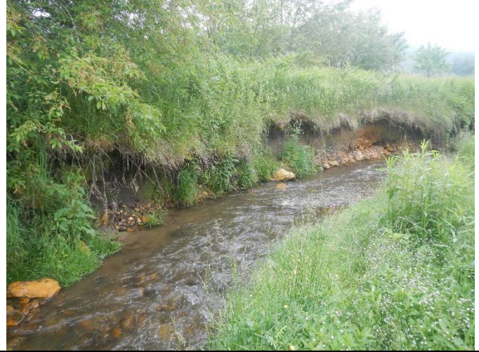
Little Pine Creek, just upstream of Glade Creek School Road bridge. Eroded bend. 06/2013
