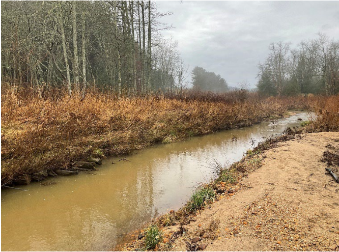
LPC Reach 1 STA 100+50 – Phase II left bank repaired with geolift and toe wood added, looking downstream (12/7/2022)
