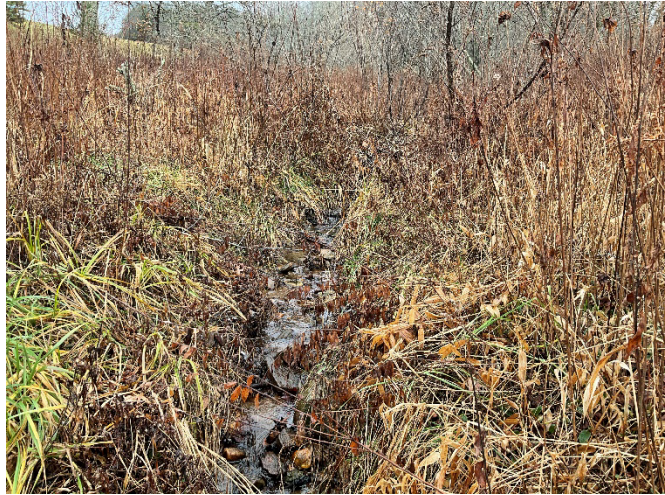
UT2B STA 505+20 – Phase III constructed riffle material added and headcut repaired, looking upstream (12/7/2022)
