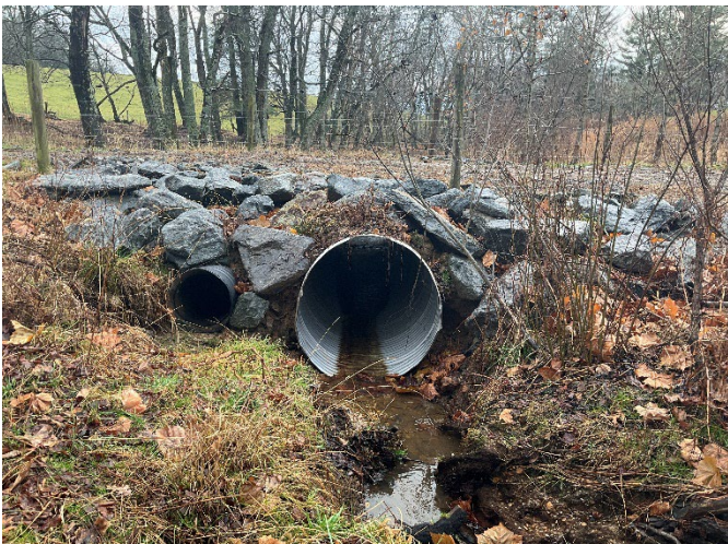
UT2 Reach 1 (Upper) STA 308+50 – Phase III repaired crossing inlet by replacing with 48" culvert, looking downstream (12/7/2022)
