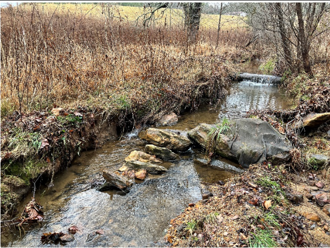
UT2 Reach 2 STA 337+50 – Right bank scour around rock vane structure, looking upstream (12/7/2022)
