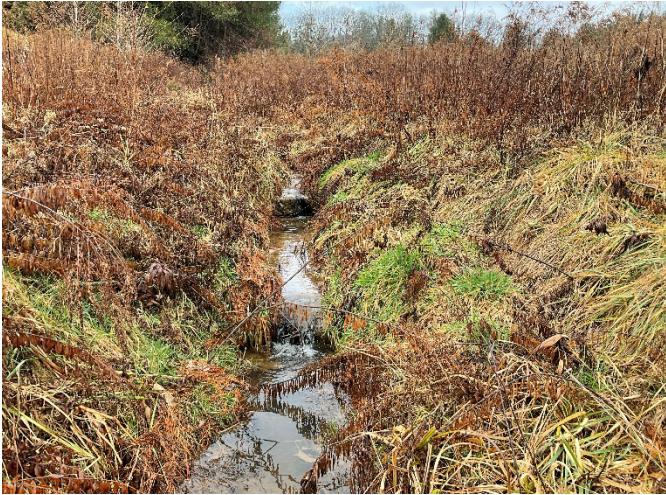
UT1 STA 198+30 – 199+00 – Phase III filter fabric added to repair piping, looking upstream (12/7/2022)
