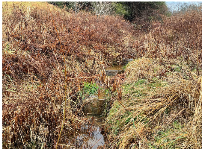
UT1 STA 198+00 – 198+30 – Phase III headcut repaired by installing rock step pools, looking upstream (12/7/2022)
