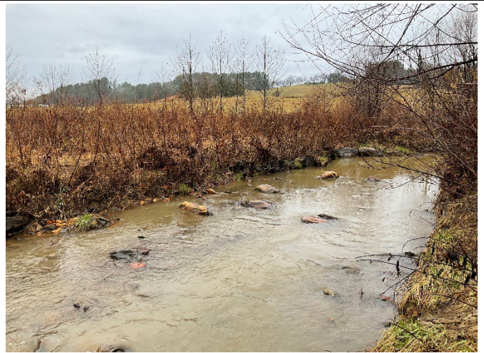
LPC Reach 2a STA 121+50 – Phase II constructed riffle and right bank repaired, looking upstream (12/7/2022)
