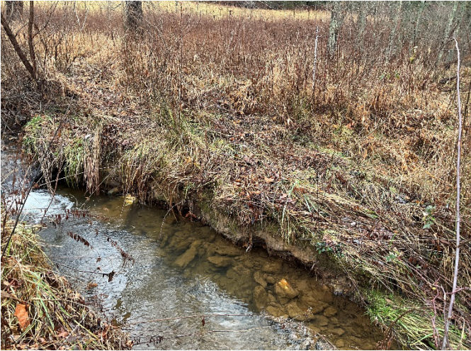
UT2 Reach 2 STA 334+40 – Left bank scour, looking upstream (12/7/2022)
