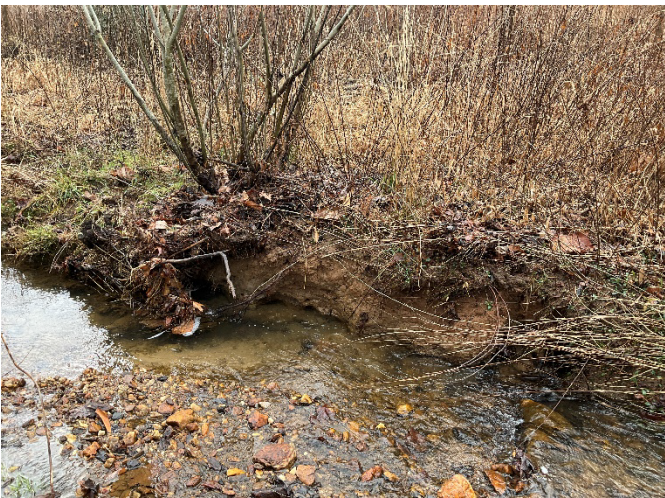
UT2 Reach 2 STA 338+30 – Right bank scour, looking at right bank (12/7/2022)
