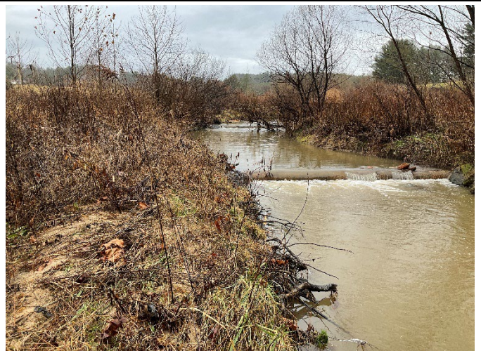
LPC Reach 2b STA 124+50 – Phase III roller log repaired and right bank geolift with toe wood, looking upstream (12/7/2022)
