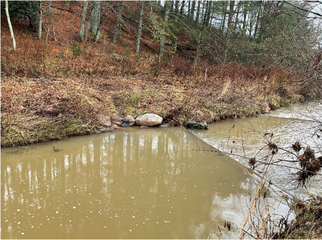
LPC Reach 2b STA 125+50 – Phase III wetland GG outlet repaired with step pool outlets, looking downstream (12/7/2022)
