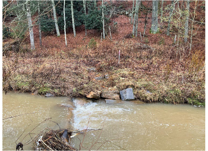
LPC Reach 2b STA 125+75 – Phase III wetland GG outlet repaired with step pool outlets, looking at left bank (12/7/2022)
