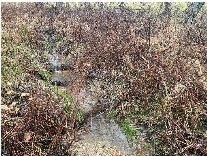
UT2 Reach 1 (Upper) STA 303+16 – Phase III filter fabric installed to repair piping log roller, looking upstream (12/7/2022)
