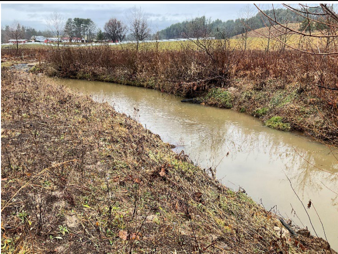
LPC Reach 2a STA 123+00 – Phase III lunker log removed, and left bank repaired, looking downstream (12/7/2022)
