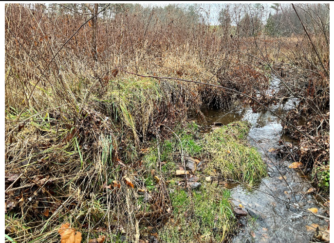
UT2 Reach 2 STA 334+10 – Right bank scour, looking upstream (12/7/2022)
