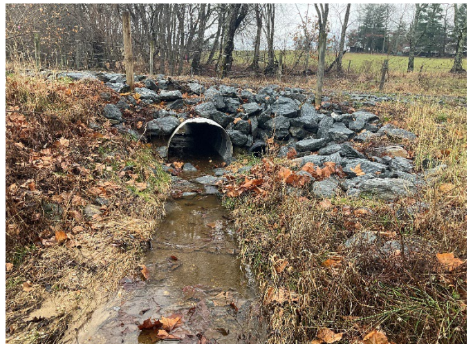
UT2 Reach 1 (Upper) STA 308+75 – Phase III repaired culvert outlet, stone added to plunge pool, looking upstream (12/7/2022)
