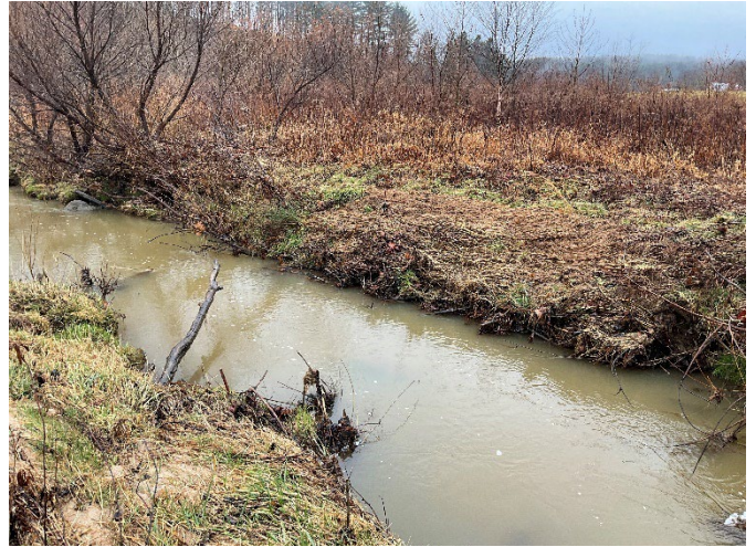
LPC Reach 2a STA 118+00 – Phase III right bank repaired with geolift and toe wood, looking downstream (12/7/2022)
