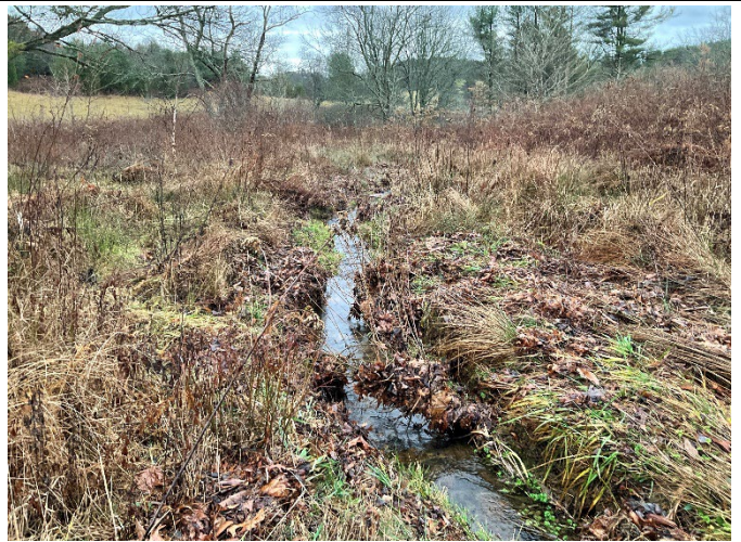
UT2A STA 430+50 – Phase I repair area stone and log step pool added, looking downstream (12/7/2022)
