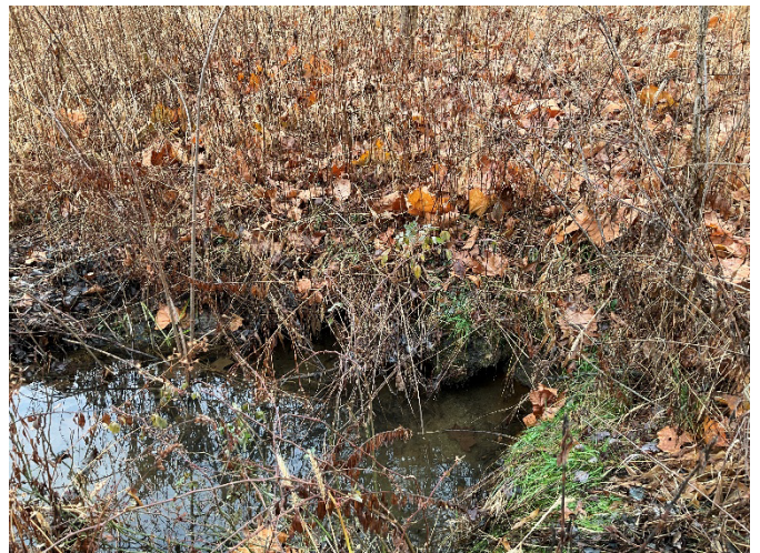
UT2B STA 504+20 – Right bank scour, looking at right bank (12/7/2022)
