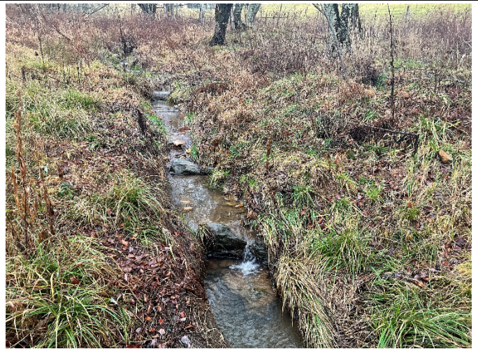
UT2 Reach 1 (Upper) STA 303+80 – 304+20 – Phase III rock cross vanes installed and right bank repaired, looking upstream (12/7/2022)
