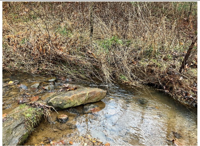
UT2 Reach 2 STA 338+00 – Left bank scour, looking at left bank (12/7/2022)
