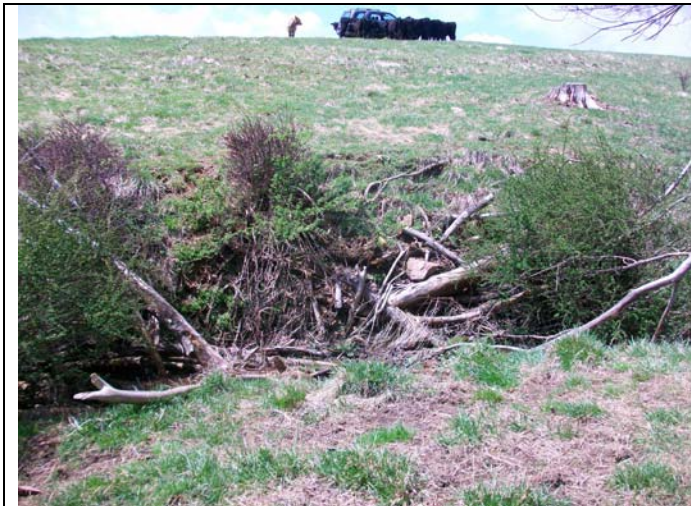
UT2A, upstream reach – debris piled in channel, cattle in field
