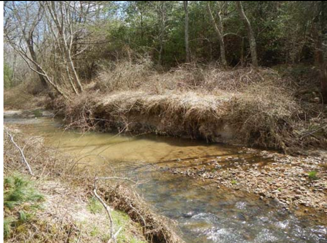
Little Pine, Reach 1 – bank erosion through wooded parcel
