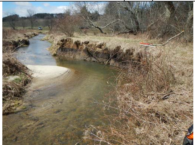
Little Pine, Reach 1 – erosion in meander bend
