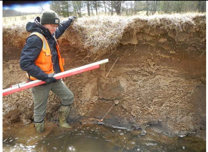
Little Pine, Reach 1 – bank erosion on pastured parcel
