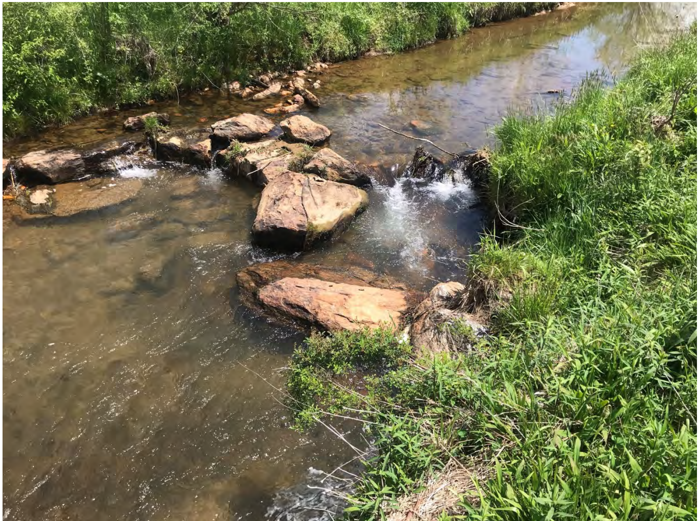
Failing J-hook structure along Little Pine Creek
