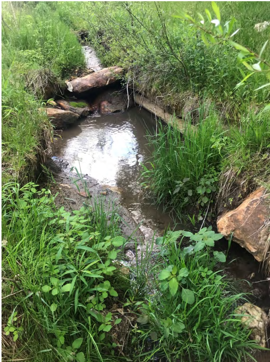
Piping structure and bank instability
