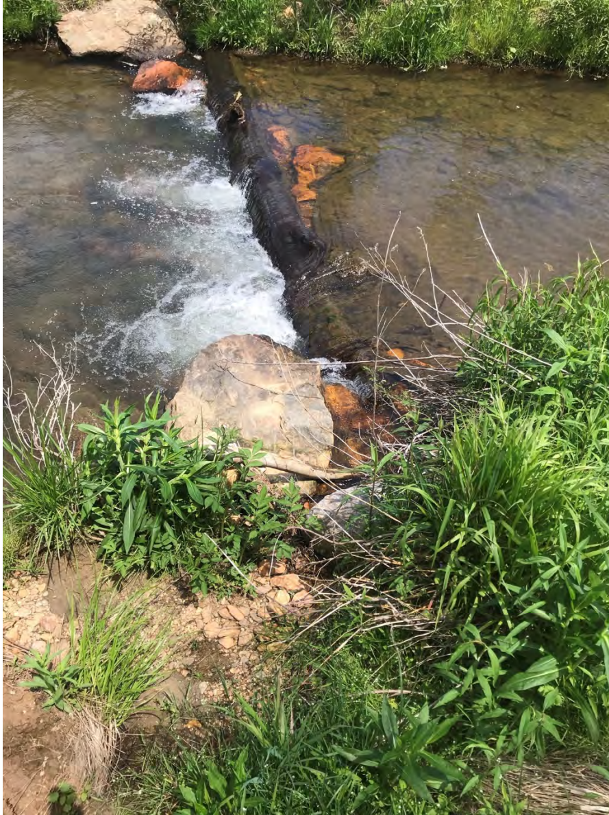
Bank erosion at log step on Little Pine Creek
