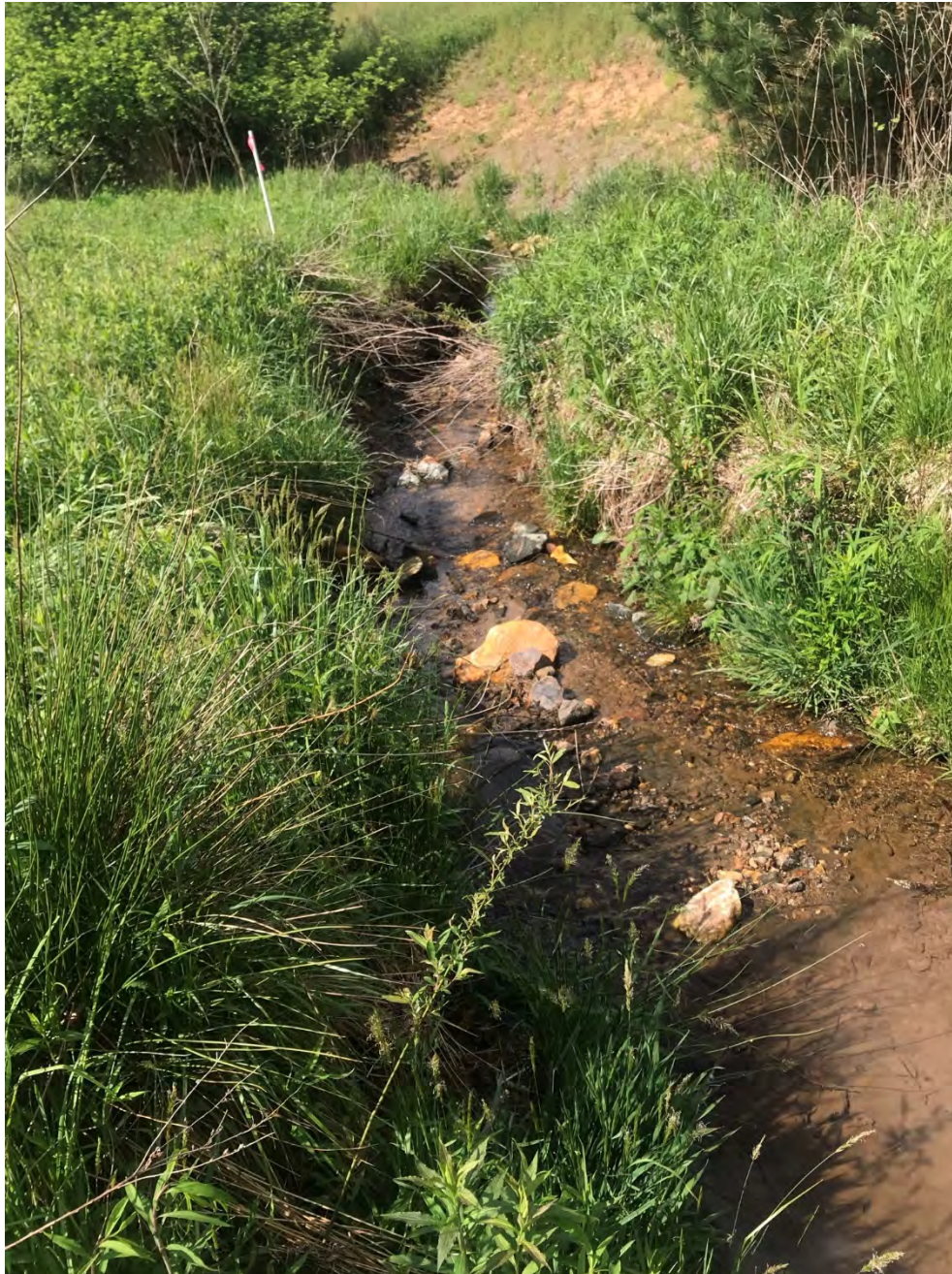
Bank erosion along UT2A
