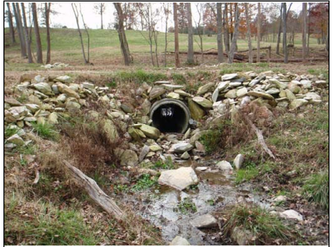
Crossing at UT2 – to be improved
