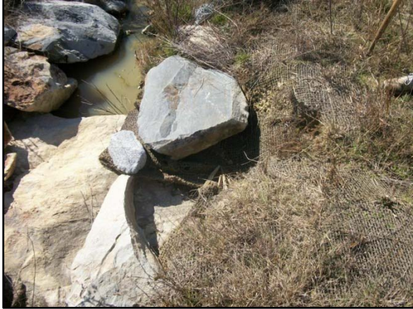
Structural Problem Area-1 Shifted Bank Armor of Boulder Step Station – 13+50
