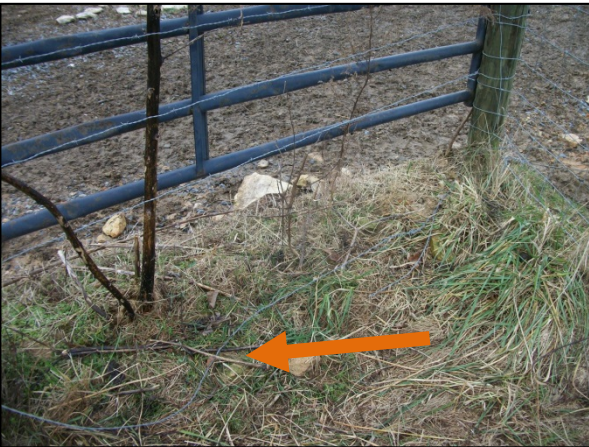
SPA 2 – Fence Repair Needed on UT2 Crossing
