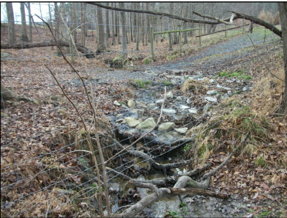
SPA 3 – Ford Crossing is Washing Out
