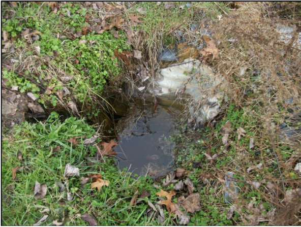
SPA 4 – Culvert & Sinkhole Repair Needed on UT3 Crossing
