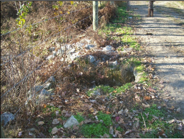
SPA 1 – Sink Hole Developing at Culvert on UT2 Crossing
