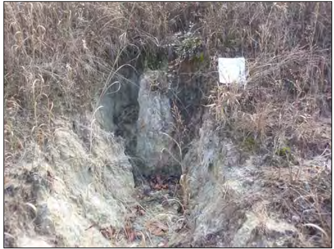
11/21/2013 MY04 – slope erosion (Stationing 55+40)
