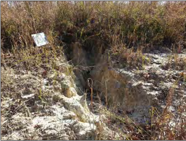
11/5/2012 MY03– slope erosion (Stationing 55+40)
