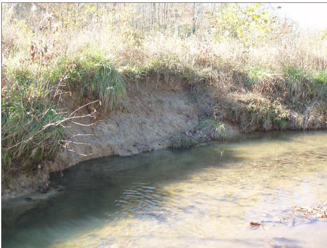
Bank Erosion at Station 13+80 11/10/14 – MY05
