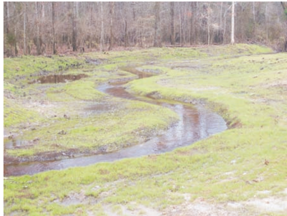
Looking upstream at upper reach of the Eastern Tributary where a floodplain bench was excavated to encourage overbank flooding.
