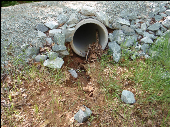
Evidence of scour and debris deposition in floodplain overflow pipe at crossing in upper R3 (photo: 4/18/19)
