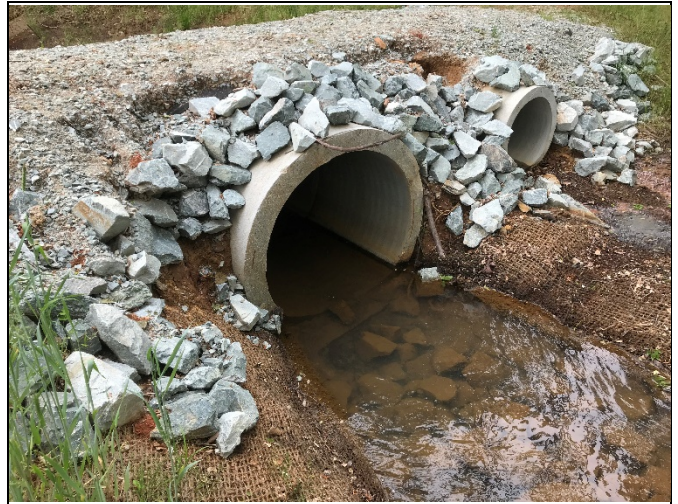
Pipe crossing collapse on R3 (downstream side) at Station 16+50
