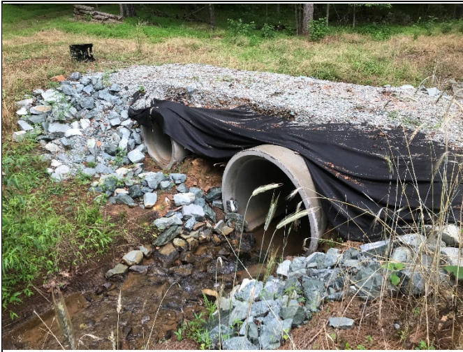
Pipe crossing collapse on R3 (upstream side) at Station 16+20
