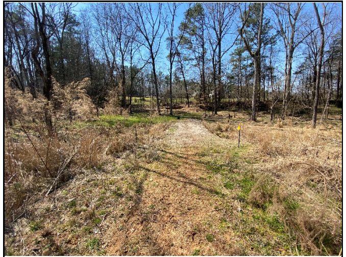
Stable pipe crossing on R3 at Station ~16+30 (3/11/21)
