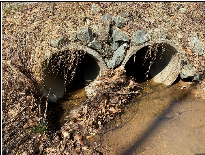
Pipes at crossing at top of R3 at Station 10+00 (3/11/21)
