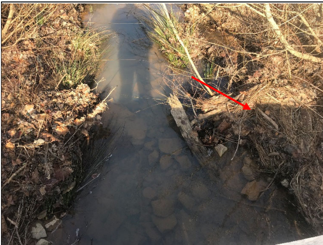
Debris jam/wrack line near crossing (photo from 3/15/22)
