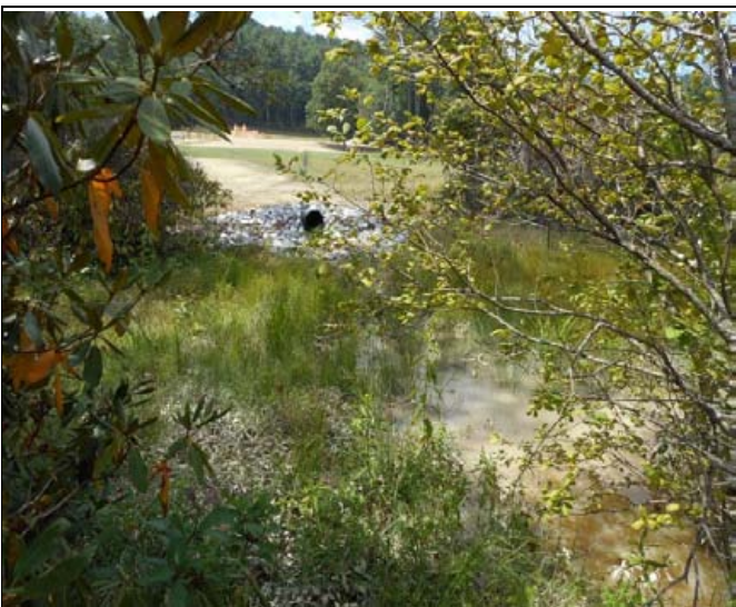
Photo 6. Encroachment by pipe installation, showing opening with standing water and silt on vegetation.
