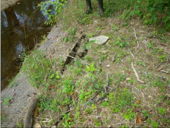
Photo 2. Bank Scour – Station 24+90, Small hole on the floodplain developed from water standing over woody debris of geolift.
