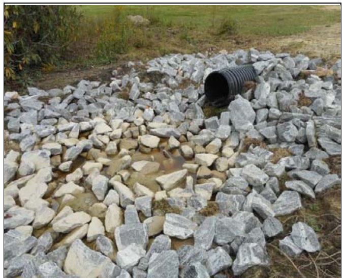
Photo 7. Encroachment by pipe installation showing outlet and riprap apron.
