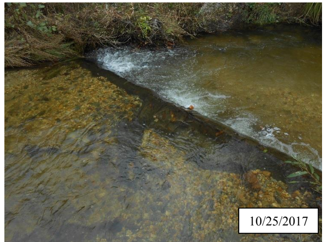
Photo 4. CPA 2-2 – Station 2+00, Piping structure was repaired in May 2017. Fabric was replaced and substrate was replaced upstream of log structure.
