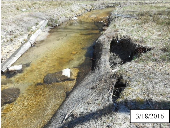
Photo 5. CPA 2-3 – Station 4+60, small area of bank scour caused by flooding of December and January 2016.
