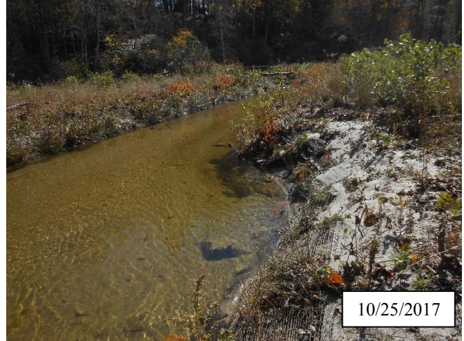
Photo 12. CPA 2-6 – Station 27+00, bank scour area was regraded, matting was reinstalled, and herbaceous vegetation was transplanted in May 2017. Livestakes were installed in October 2017.
