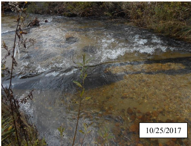
Photo 15. CPA 3-3 – Station 14+75, piping of log structure after the fabric sealing this structure tore in 2017. This structure will be repaired in 2018.
