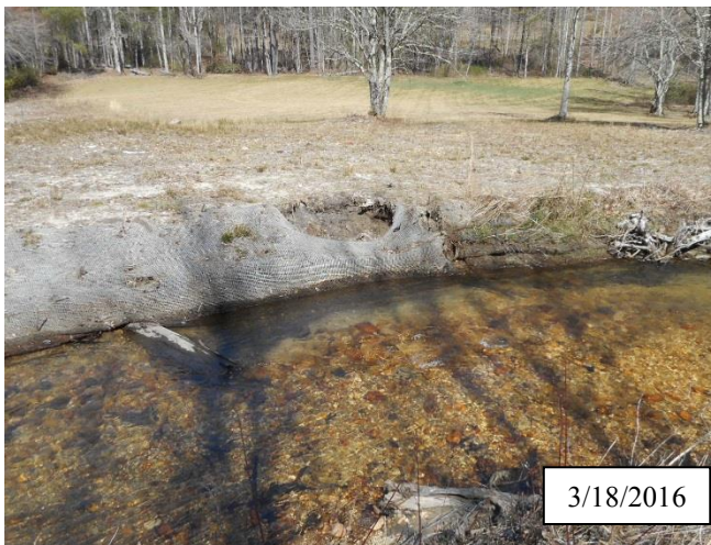
Photo 9. CPA 2-5 – Station 26+60, small area of bank scour caused by flooding of December and January 2016.
