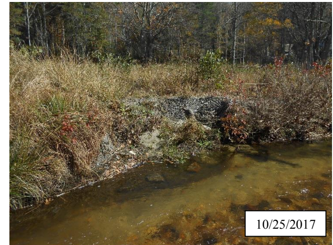
Photo 10. CPA 2-5 – Station 26+60, bank scour area was regraded, matting was reinstalled, and herbaceous vegetation was transplanted in May 2017. Livestakes were installed in October 2017.
