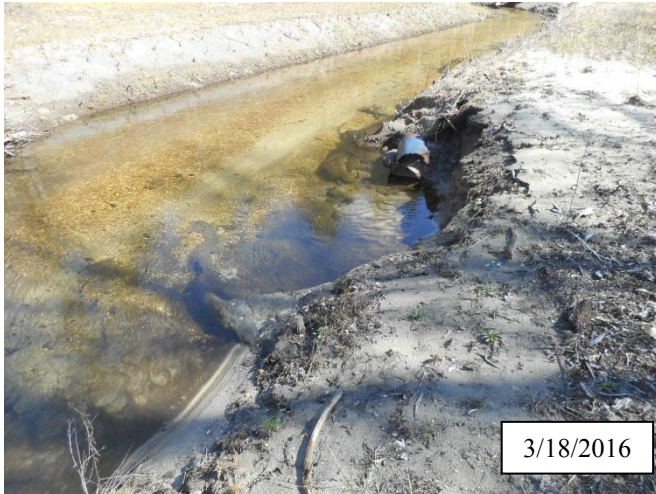
Photo 11. CPA 2-6 – Station 27+00, small area of bank scour caused by flooding of December and January 2016.
