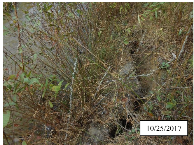
Photo 14. CPA 3-2 – Station 21+00, small bank slump area (approx. 6 ft.) along left bank of main stem. Will be monitored to see if the bank stabilizes in MY4
