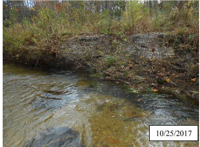
Photo 6. CPA 2-3 – Station 4+60, bank scour area was regraded, matting was reinstalled, and herbaceous vegetation was transplanted in May 2017. Livestakes were installed in October 2017.
