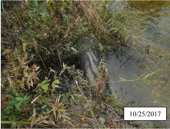
Photo 17. CPA 3-5 – Station UT8 00+40, piping of log structure on UT-8 near the confluence of UT-8 and Logan Creek
