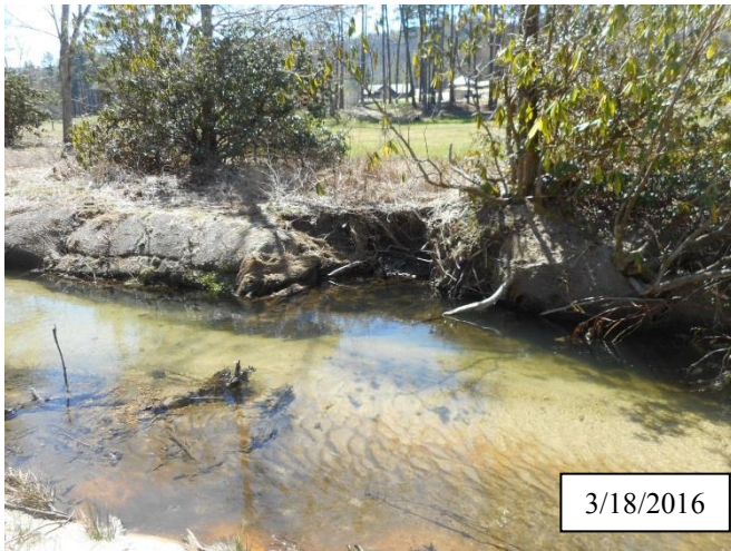
Photo 7. CPA 2-4 – Station 11+70, small area of bank scour caused by flooding of December and January 2016.
