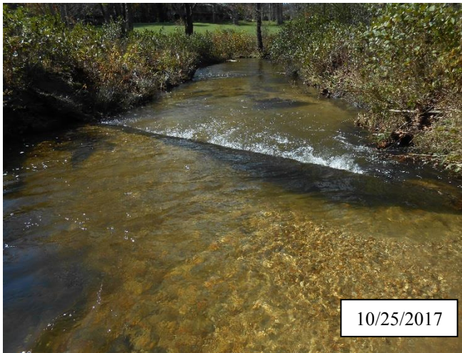
Photo 13. CPA 3-1 – Station 23+75, piping of log structure after the fabric sealing this structure tore in 2017. This structure will be repaired in 2018.
