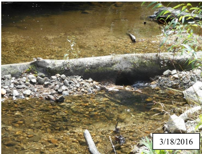
Photo 3. CPA 2-2 – Station 2+00, Piping of log structure after the fabric sealing this structure tore during flooding of December and January.
