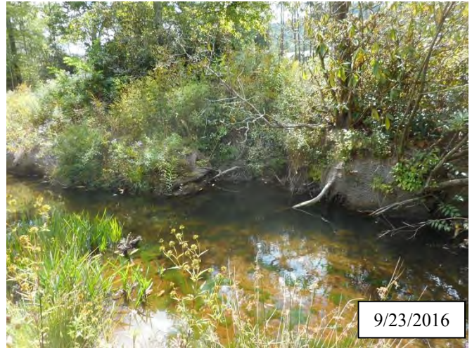
Photo 11. CPA 2-4 – Station 11+70, scour area noted in MY2 has stabilized for the most part. Livestakes were planted in the scour area as well as the bank downstream of the problem area in October 2017.
