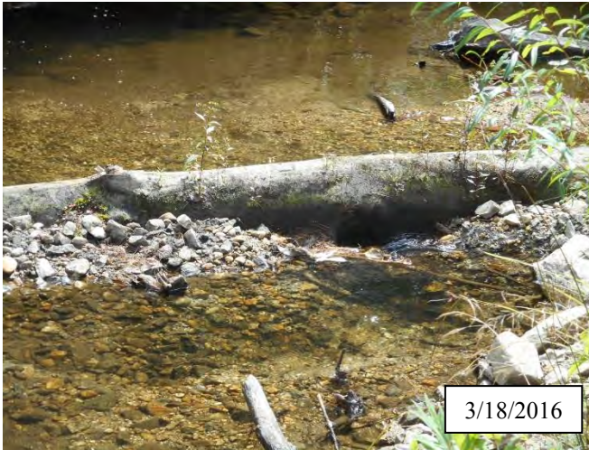
Photo 4. CPA 2-2 – Station 2+00, Piping of log structure after the fabric sealing this structure tore during flooding of December and January 2016.
