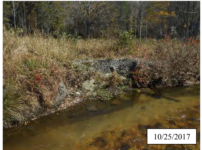
Photo 14. CPA 2-5 – Station 26+60, bank scour area was regraded, matting was reinstalled, and herbaceous vegetation was transplanted in May 2017. Livestakes were installed in October 2017.
