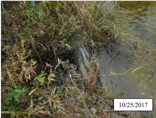
Photo 27. CPA 3-5 – Station UT8 00+40, piping of log structure on UT-8 near the confluence of UT-8 and Logan Creek. Hand repairs will be made to CPA 3-5 during MY5.
