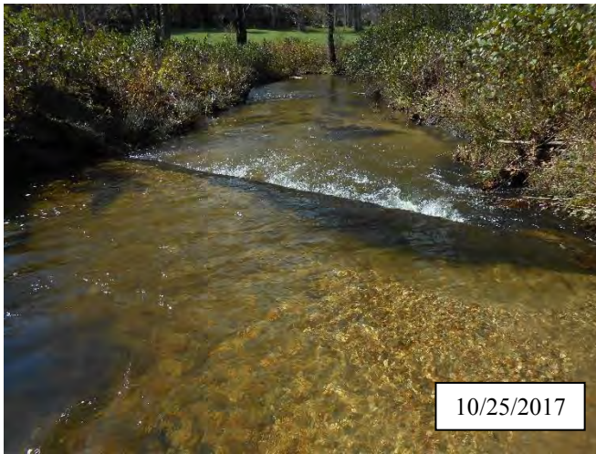
Photo 19. CPA 3-1 – Station 23+75, piping of log structure after the fabric sealing this structure tore in 2017.
