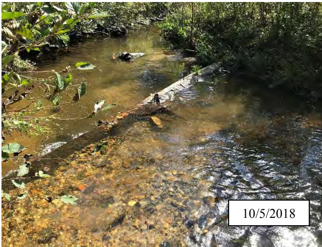
Photo 6. CPA 2-2 – Log structure that was repaired in 2017 has remained stable and is no longer piping.
