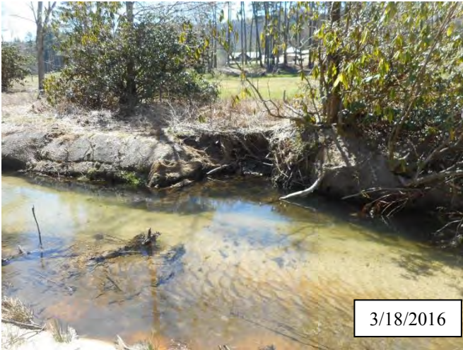
Photo 10. CPA 2-4 – Station 11+70, small area of bank scour caused by flooding of December and January 2016.
