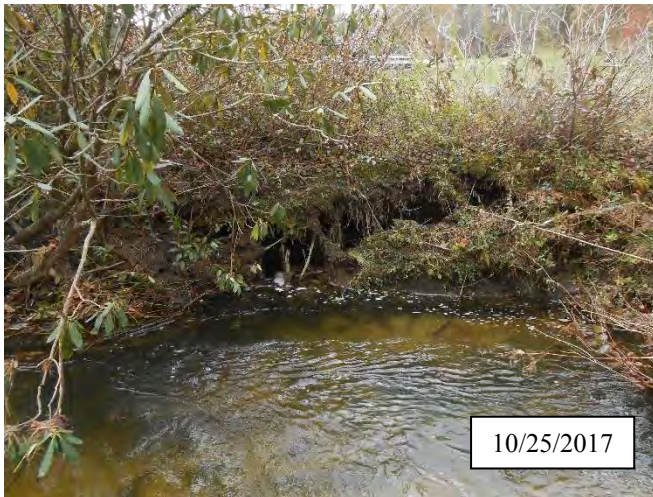
Photo 25. CPA 3-4 – Station 11+50, small bank slump (approx. 8 ft.) along right bank of main stem.
