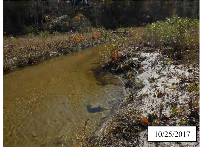
Photo 17. CPA 2-6 – Station 27+00, bank scour area was regraded, matting was reinstalled, and herbaceous vegetation was transplanted in May 2017. Livestakes were installed in October 2017.
