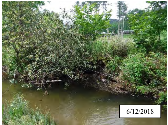
Photo 26. CPA 3-4 – Station 11+50, slump area has not stabilized but has not worsened in 2018. Will continue to monitor in MY5.
