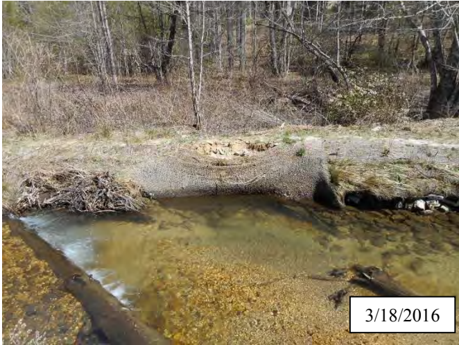
Photo 1. CPA 2-1 – Station 2+10, small area of bank scour caused by flooding of December and January 2016.
