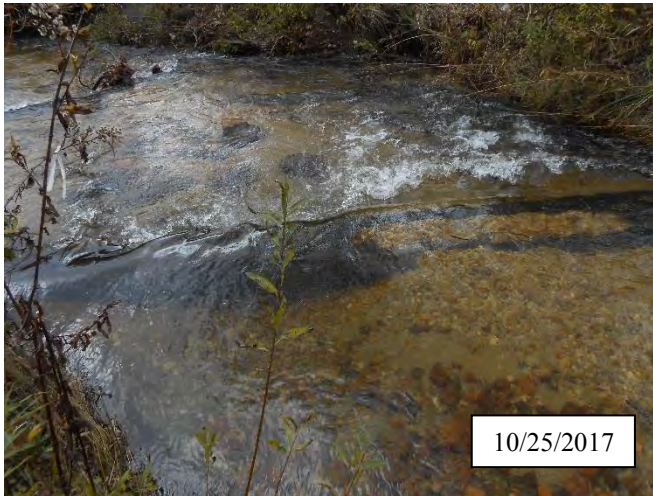
Photo 23. CPA 3-3 – Station 14+75, piping of log structure after the fabric sealing this structure tore in 2017.
