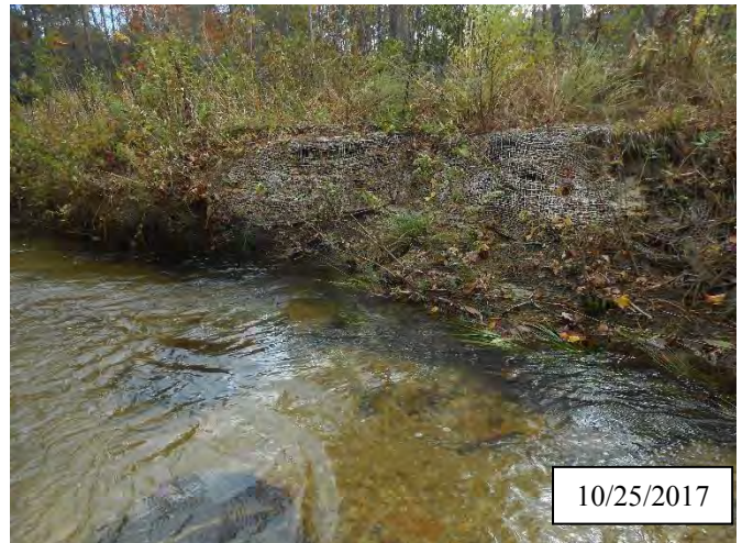
Photo 8. CPA 2-3 – Station 4+60, bank scour area was regraded, matting was reinstalled, and herbaceous vegetation was transplanted in May 2017. Livestakes were installed in October 2017.
