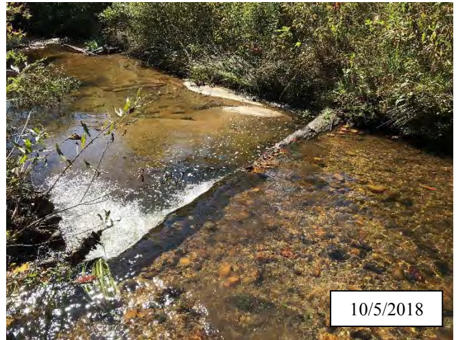
Photo 24. CPA 3-3 – Station 14+75, piping log structure has stabilized and is no longer piping in 2018.
