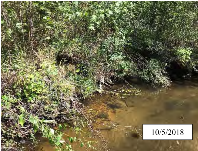
Photo 3. CPA 2-1 – Scour area has stabilized and is no longer eroding after repairs were made in 2017.
