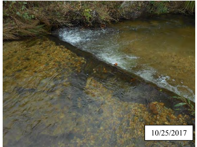
Photo 5. CPA 2-2 – Station 2+00, Piping structure was repaired in May 2017. Fabric was replaced and substrate was replaced upstream of log structure.
