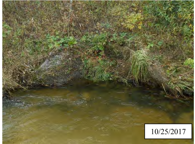
Photo 2. CPA 2-1 – Station 2+10, same area as shown in photo 1 during October 2017 with vegetation stabilizing site. Bank was graded, matting was reinstalled, and live stakes were added during October 2017.
