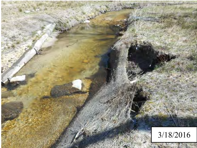
Photo 7. CPA 2-3 – Station 4+60, small area of bank scour caused by flooding of December and January 2016.
