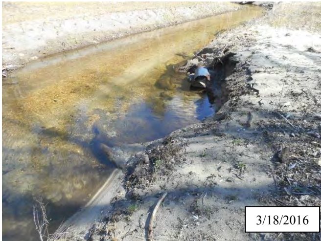
Photo 16. CPA 2-6 – Station 27+00, small area of bank scour caused by flooding of December and January 2016.
