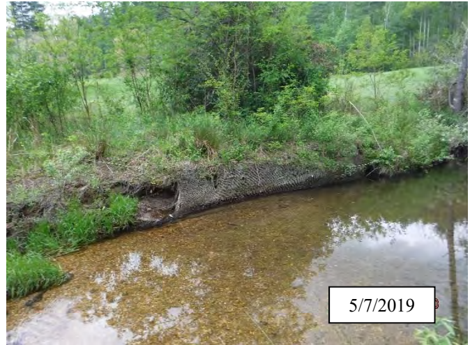
Photo 16. CPA 2-4 – Station 11+70, Bank maintained not completely stable but improving with growing vegetation in 2019
