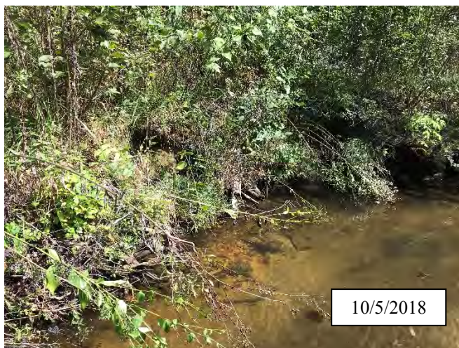
Photo 3. CPA 2-1, Scour area has stabilized and is no longer eroding after repairs were made in 2017.
