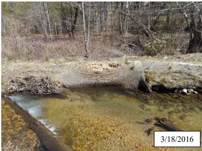
Photo 1. CPA 2-1, Station 2+10, small area of bank scour caused by flooding of December and January.
