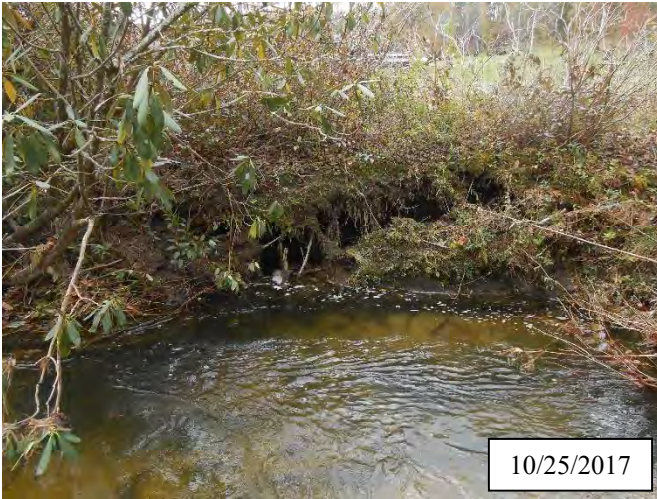
Photo 35. CPA 3-4 – Station 11+50, small bank slump (approx. 8 ft.) along right bank of main stem.
