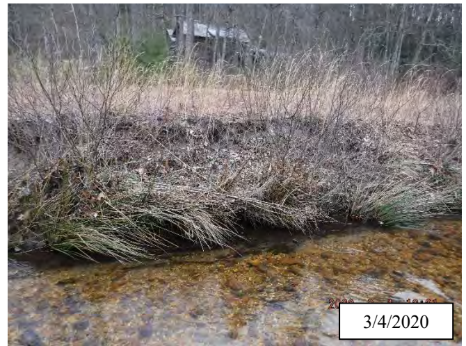
Photo 20. CPA 2-5 – Station 26+60, Scour area stabilized with vegetation in 2019, late winter photo (3-2020).
