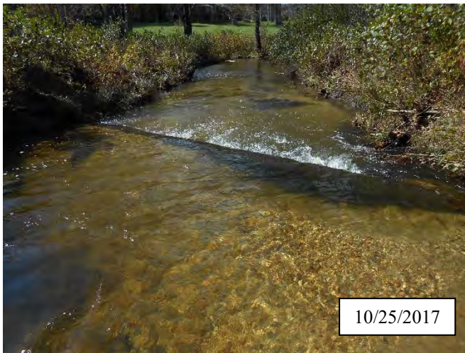
Photo 26. CPA 3-1 – Station 23+75, piping of log structure after the fabric sealing this structure tore in 2017.
