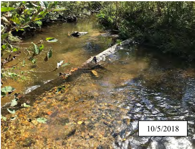
Photo 7. CPA 2-2 – Log structure that was repaired in 2017 has remained stable and is no longer piping.
