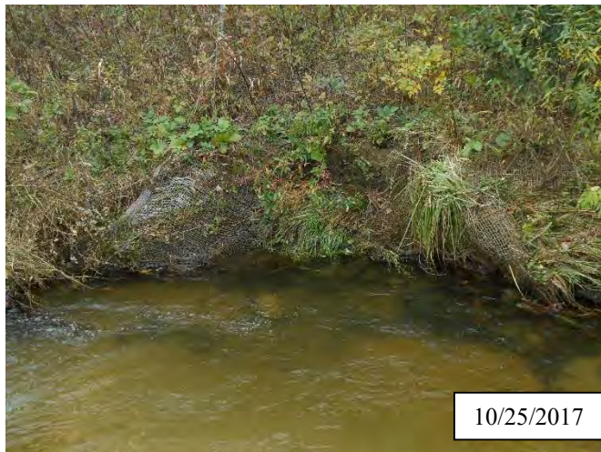
Photo 2. CPA 2-1, Station 2+10, same area as shown in photo 1, with vegetation stabilizing site. Bank was graded, matting was reinstalled, and live stakes were added during October 2017.
