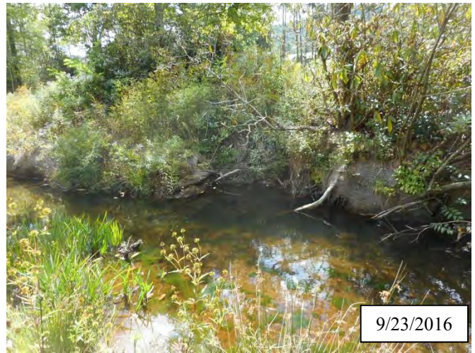
Photo 14. CPA 2-4 – Station 11+70, scour area noted in MY2 has stabilized for the most part. Livestakes were planted in the scour area as well as the bank downstream of the problem area in October 2017.
