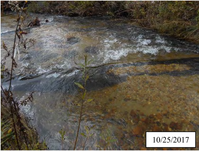
Photo 32. CPA 3-3 – Station 14+75, piping of log structure after the fabric sealing this structure tore in 2017.
