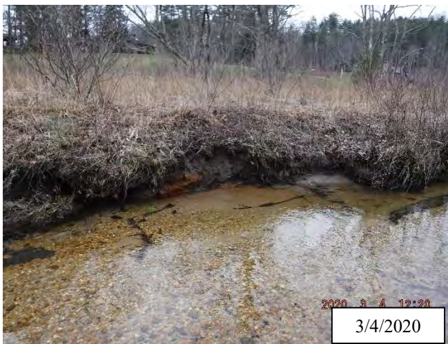
Photo 25. CPA 2-6 – Station 27+00, scour area vegetated and stable, some bare bank late winter (3-2020).
