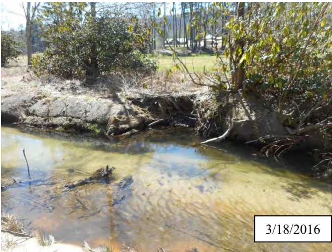
Photo 13. CPA 2-4 – Station 11+70, small area of bank scour caused by flooding of December and January 2016.
