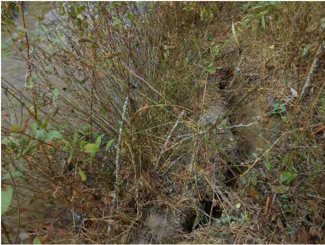
Photo 29. CPA 3-2 – Station 21+00, small bank slump area (approx. 6 ft.) along left bank of main stem.
