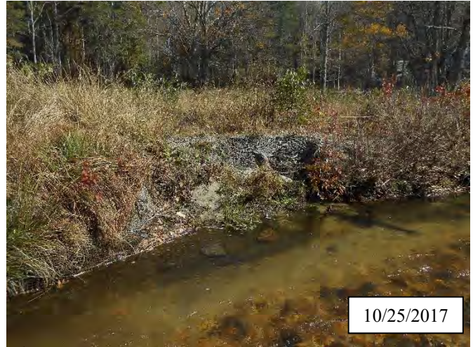
Photo 18. CPA 2-5 – Station 26+60, bank scour area was regraded, matting was reinstalled, and herbaceous vegetation was transplanted in May 2017. Livestakes were installed in October 2017.
