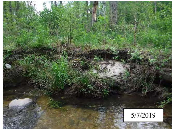
Photo 12. CPA 2-3 – Station 4+60, bank scour area maintaining vegetation but still some signs it is not completely stable.
