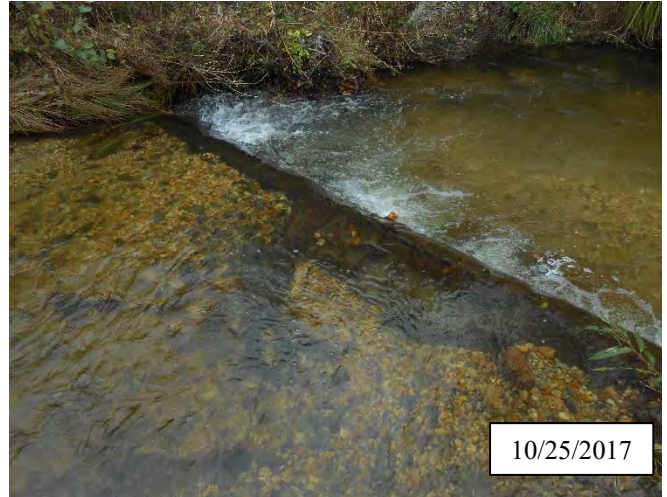
Photo 6. CPA 2-2 – Station 2+00, Piping structure was repaired in May 2017. Fabric was replaced and substrate was replaced upstream of log structure.
