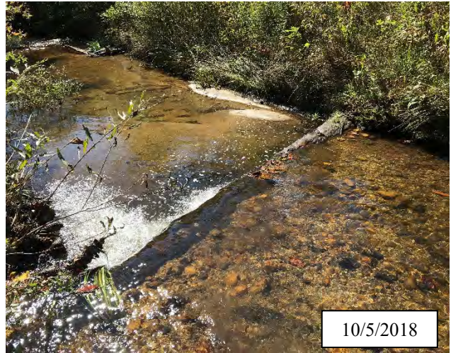
Photo 33. CPA 3-3 – Station 14+75, piping log structure has stabilized and is no longer piping in 2018.
