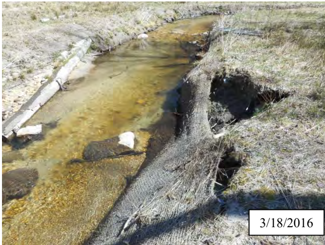
Photo 9. CPA 2-3 – Station 4+60, small area of bank scour caused by flooding of December and January 2016.
