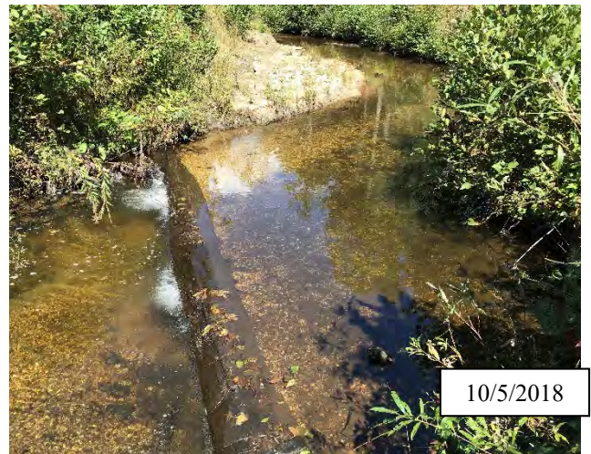
Photo 27. CPA 3-1 – Log structure has stabilized and is no longer piping.
