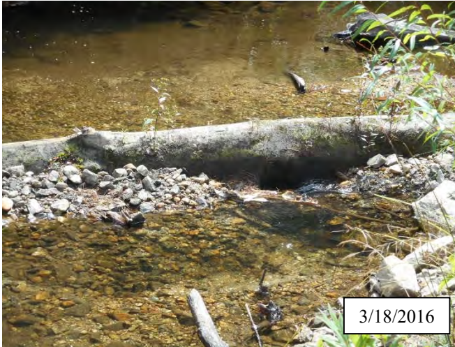
Photo 5. CPA 2-2 – Station 2+00, Piping of log structure after the fabric sealing this structure tore during flooding of December and January.
