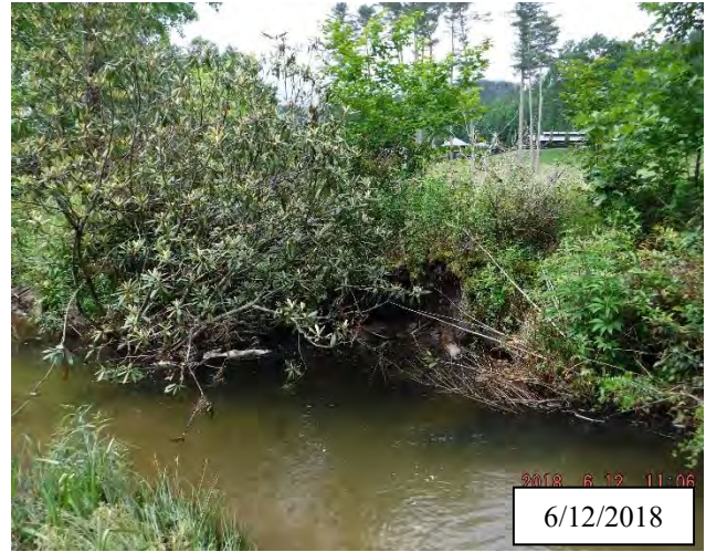
Photo 36. CPA 3-4 – Station 11+50, slump area has not stabilized but has not worsened in 2018.
