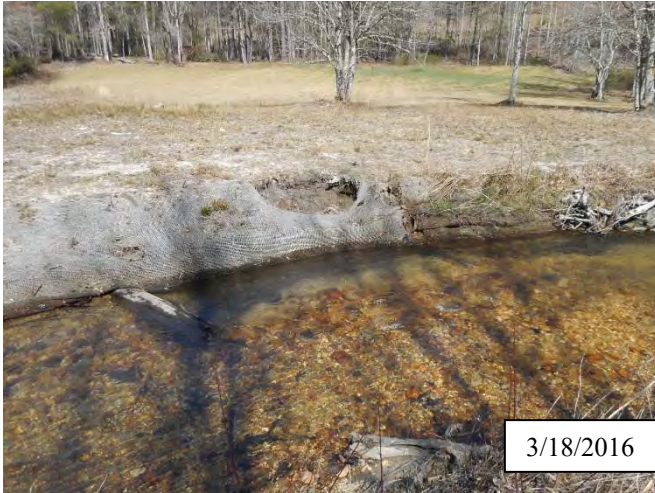
Photo 17. CPA 2-5 – Station 26+60, small area of bank scour caused by flooding of December and January 2016.
