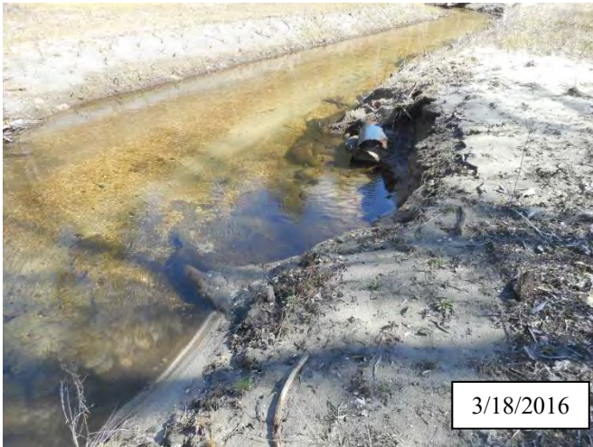
Photo 21. CPA 2-6 – Station 27+00, small area of bank scour caused by flooding of December and January 2016.
