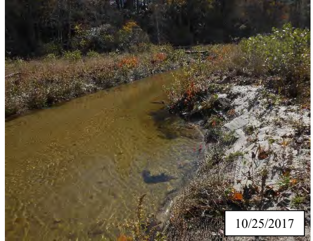
Photo 22. CPA 2-6 – Station 27+00, bank scour area was regraded, matting was reinstalled, and herbaceous vegetation was transplanted in May 2017. Livestakes were installed in October 2017.
