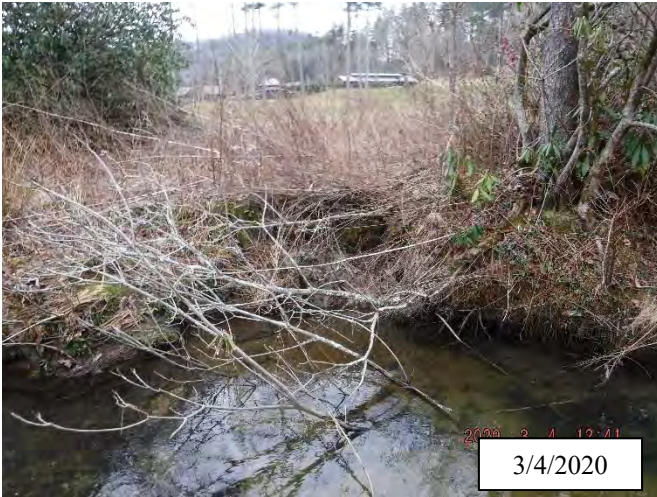
Photo 37. CPA 3-4 – Station 11+50, slump area left a gap in the bank but it is stable in late winter 2020.
