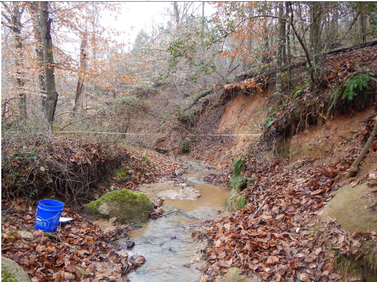
UT1 – Reach 2A. Heavy sediment load, valley wall and bank erosion near bedrock outcrop
