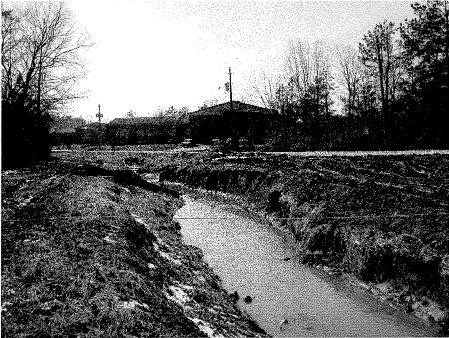
4. View of stream where Burnette Road and town maintained dirt access path to sewer lift station intersect.
